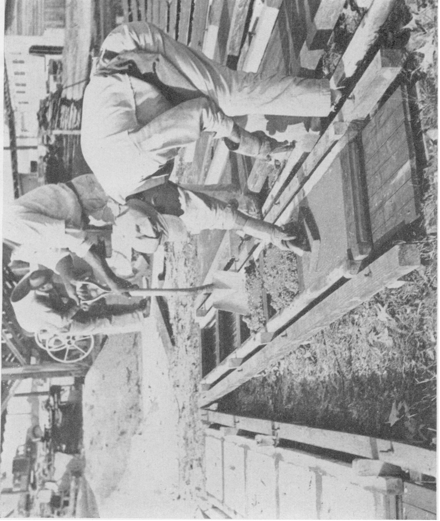
FIGURE 15.—Arrangement of slab-casting yard, showing assembled form and details of casting the slab.
