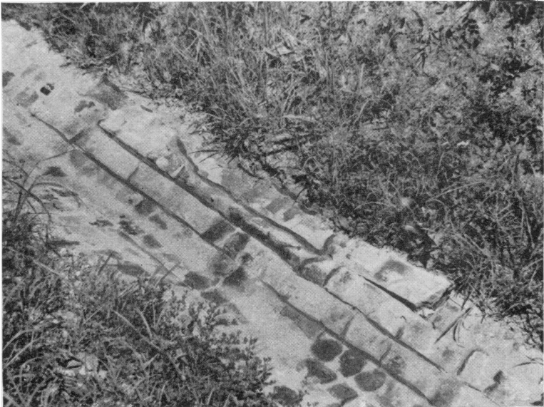
FIGURE 14.—Well-bonded brick broken away from the mother lining. Break was due to settling of backfill
