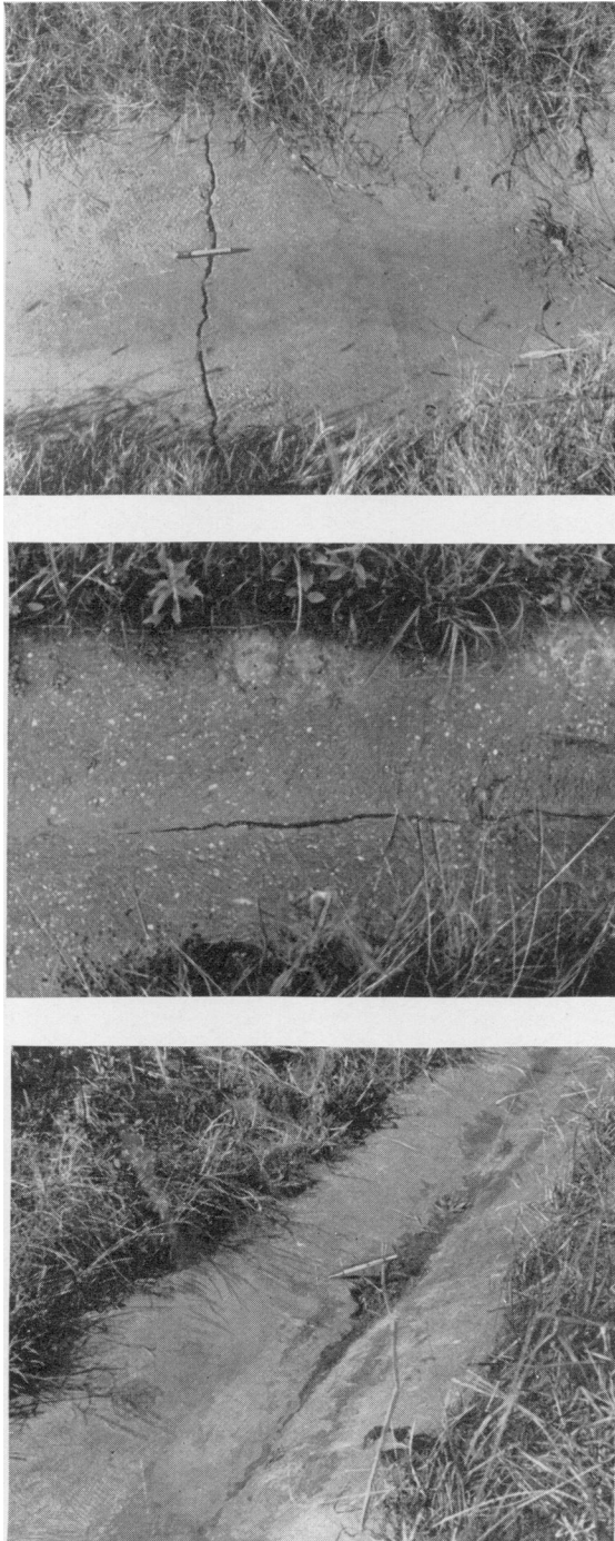
FIGURE 5.—Transverse and longitudinal cracking and holes in monolithic concrete slabs.
