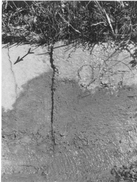
FIGURE 4.—Crack at extreme left (arrow) caused by compression resulting from lack of expansion joint between the two sections. Dark line along ends of slabs (center) is not an opening but a shadow cast by slab on right which has "overlapped" slab on left.
