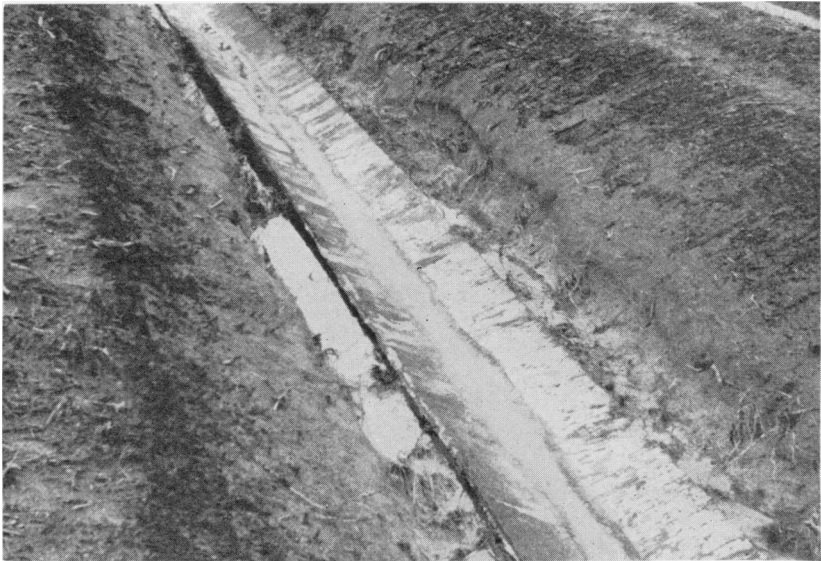
FIGURE 10.—Newly installed monolithic lining intact after being subjected to intense scouring run-off. Note destruction of freshly sodded ditchbanks.
