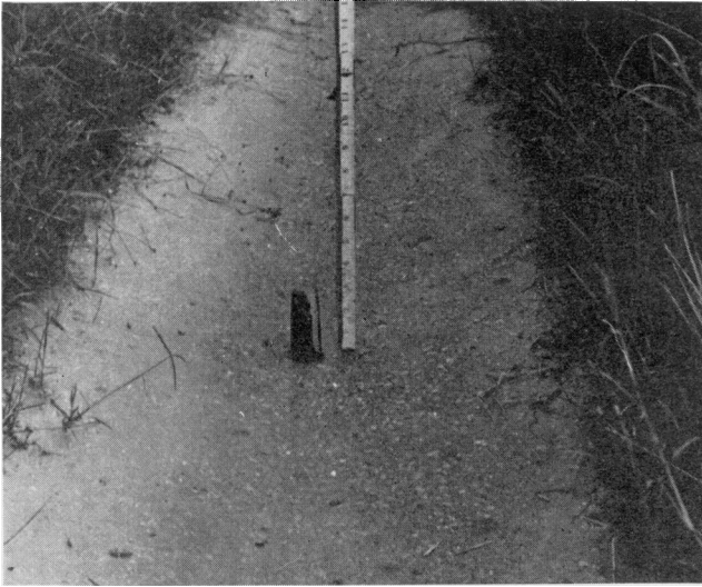
FIGURE 9.—Grade stake pushed above lining by frost action, a distance of 3 inches
