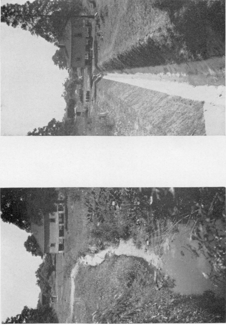
FIGURE 1.—Before and after installation of durable malaria control drainage. (Photographs by courtesy of Nelson H. Rector, Mississippi State Board of Health.)
