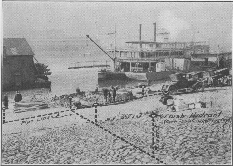
Pittsburgh levee during construction of pipe line for vessels. Dotted lines show the arrangement of pipes below the ground surface, with risers at intervals leading to hydrants flush with the surface. This use of flush hydrants avoids interference with trucking on the incline
