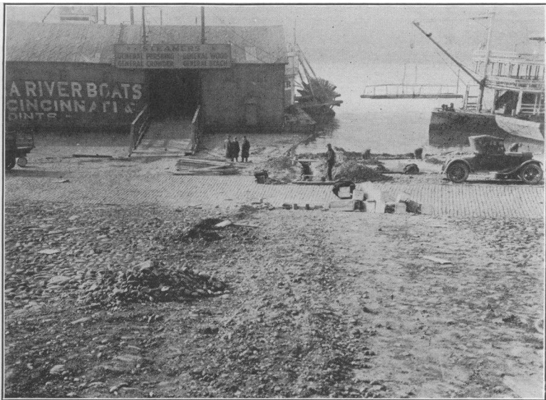
Levee at Pittsburgh, Pa., during construction of water mains for supplying city water to vessels, showing usual arrangement of wharf boat and landing stage, with steamer beyond the wharf boat
