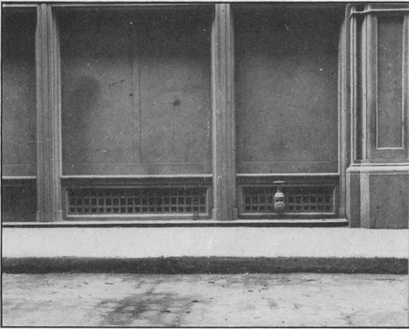
Fig. 1.—UNSCREENED BASEMENT VENTILATOR.
