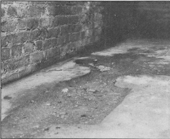
Fig. 4.—DEFECTIVE CONCRETE FLOOR IN BASEMENT, CONCRETE LAYER TOO THIN; HAS BECOME BROKEN AND NOW PERMITS BURROWING AND RAT HARBOR BENEATH.
