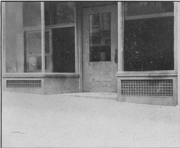
Fig. 2.—PROPERLY SCREENED BASEMENT VENTILATORS UNDER SHOW WINDOWS.
