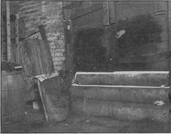
Fig. 3.—DEFECTIVE BASEMENT DOORWAY AT THE BOTTOM OF BASEMENT STAIRS.
