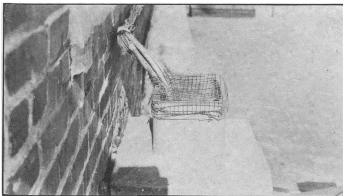
Fig. 20.—THE ROOF EXIT OF AN UNUSED CHIMNEY FLUE PROPERLY SCREENED WITH HEAVY WIRE MESH.
