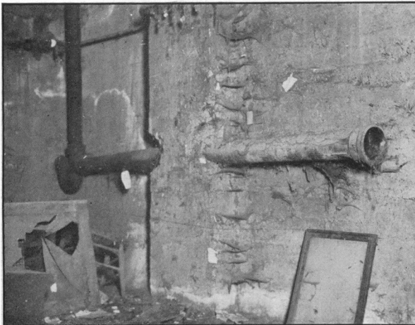
Fig. 8.—OLD ABANDONED SEWER ENTERING BASEMENT. A COMMON HIGHWAY FOR THE ENTRANCE OF RATS INTO BASEMENTS.
