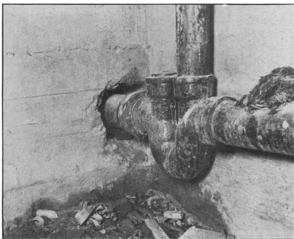
Fig. 5.—DEFECTIVE BASEMENT WALL. OPENING MADE FOR THE INSTALLATION OF HOUSE SEWAGE SYSTEM.
