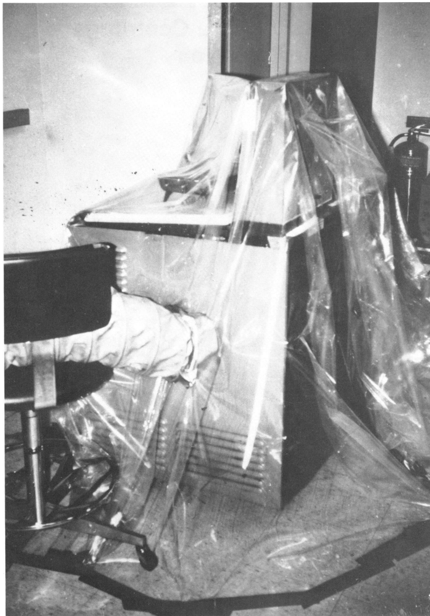
Figure 2. Exhaust connection and sealed canopy
