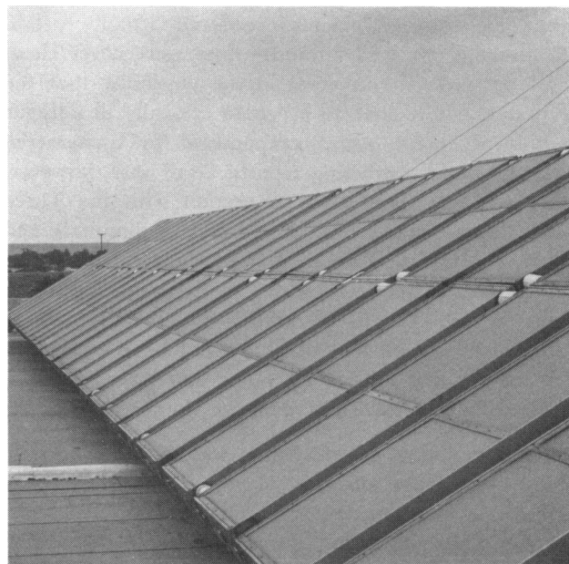
Solar collector panels
