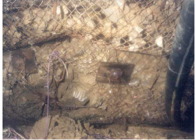
Figure 18.—Backfill failure at four-way bracket.
