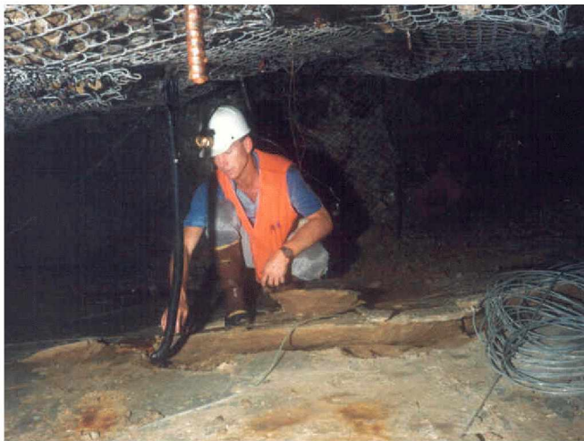
Figure 9.—Thrust-fault-type failure, November 4, 1997.
