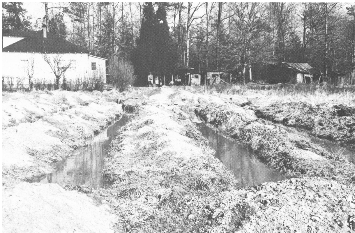
Photograph by W. J. Edmunds, Emporia, Va. Excavated drainlines for a new septic tank in wet soil which had been approved during a dry period
