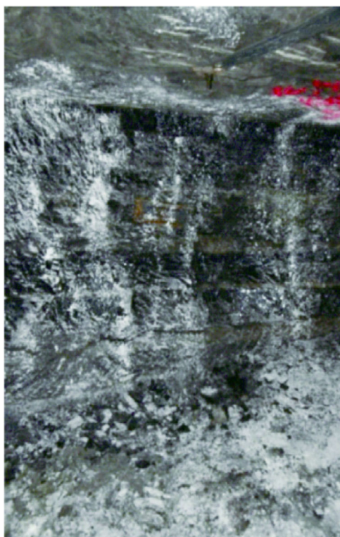
Fig. 12. Observed rib conditions at Site 2.
