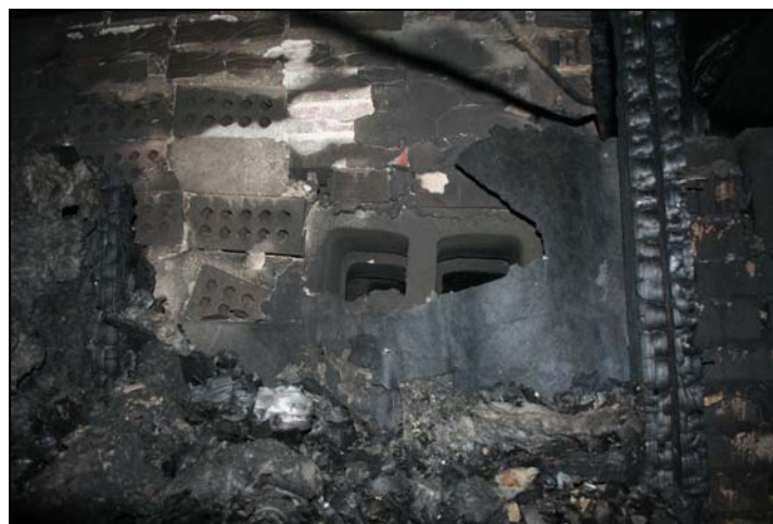
Photo 2. The picture shows the area of the brick chimney flue that was replaced with cinder blocks. The cinder blocks allowed heat and flame to impinge on the exterior wall allowing fire to spread into the attic space. (Photo courtesy of sheriff's office)
