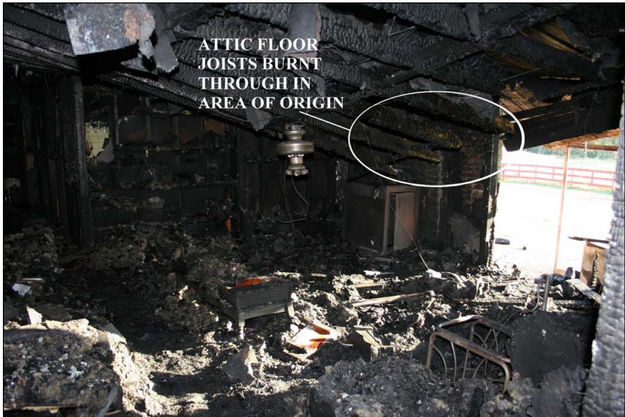
Photo 6. Fire damage to living room area before rekindle and structural collapse. (Photo courtesy of sheriff's office)
