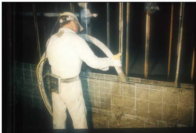
Figure 22.—Meshblock seal under construction showing the lower Meshblocks, the vertical #8 steel reinforcement bars and anchors, and placement of shotcrete.
