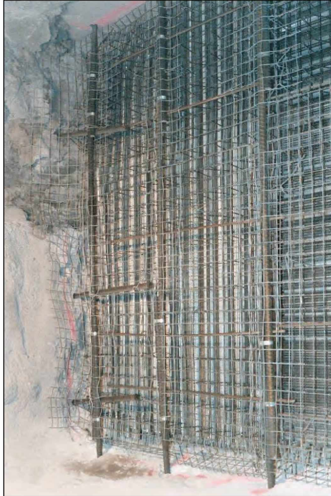
Figure 18.—Insteel 3-D seal under construction showing the rear Insteel panel with Stayform backing, one plane of vertical #8 steel reinforcement bars and anchors, the horizontal #8 steel reinforcement bar anchors, and the horizontal #3 steel reinforcement bars.
