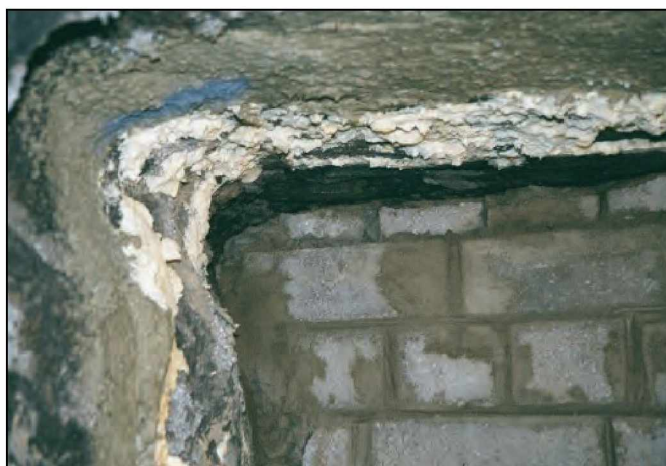
Figure 28.—In background, top of a solid-concrete-block seal showing small cut blocks and mortar filling at the seal top.
