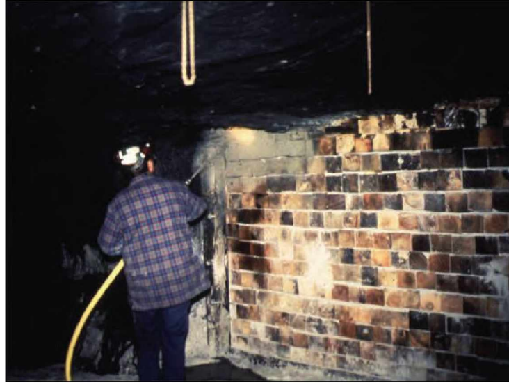
Figure 40.—Construction of a hitched wood-crib-block seal without plywood facing showing the wood crib blocks separated by a rock dust layer, the angle iron hitching around the ribs and floor only, and the final coating with an approved sealant.
