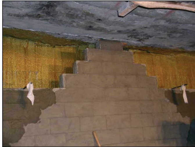
Figure 36.—Polymer and aggregate seal from MICON showing the rear dry-stacked, hollow-core concrete block wall, the partially completed front wall, a polymer coating on the inside surface of the form walls, and an approved sealant on the outside surface of the form wall.
