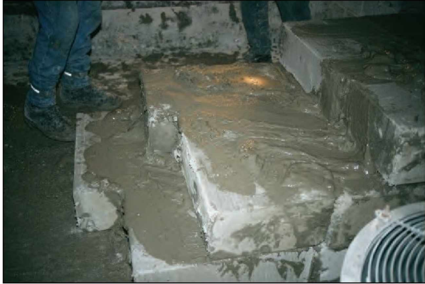
Figure 49.—Construction of a 40-in-thick Omega block seal without hitching and no center pilaster. All surfaces are coated with BlocBond mortar.
