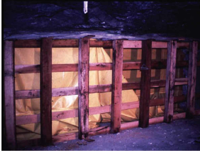
Figure 24.—Formwork for a typical pumpable seal showing the vertical posts, the horizontal boards, and the brattice liner (partially removed).
