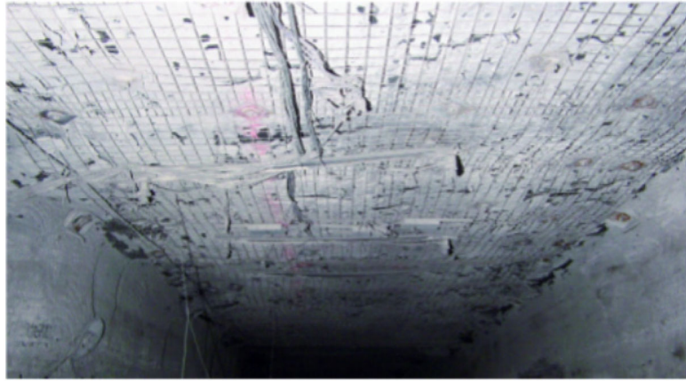
Fig. 10. Roof conditions in Entry No. 1 at the crosscut site prior to mining of the first panel.
