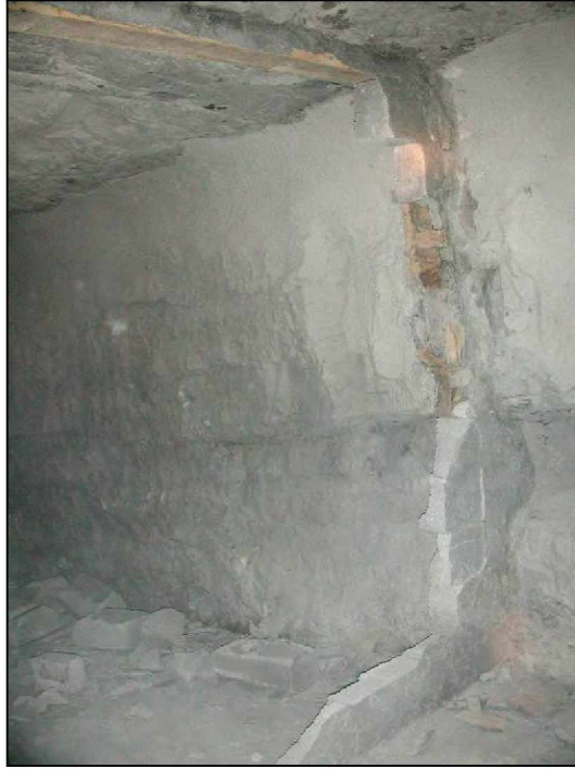
Figure 73.—Debris from the dry-stacked solid-concrete-block stopping and remaining blocks on the inby rib line in X-4 after LLEM test #462, viewed from C-drift.
