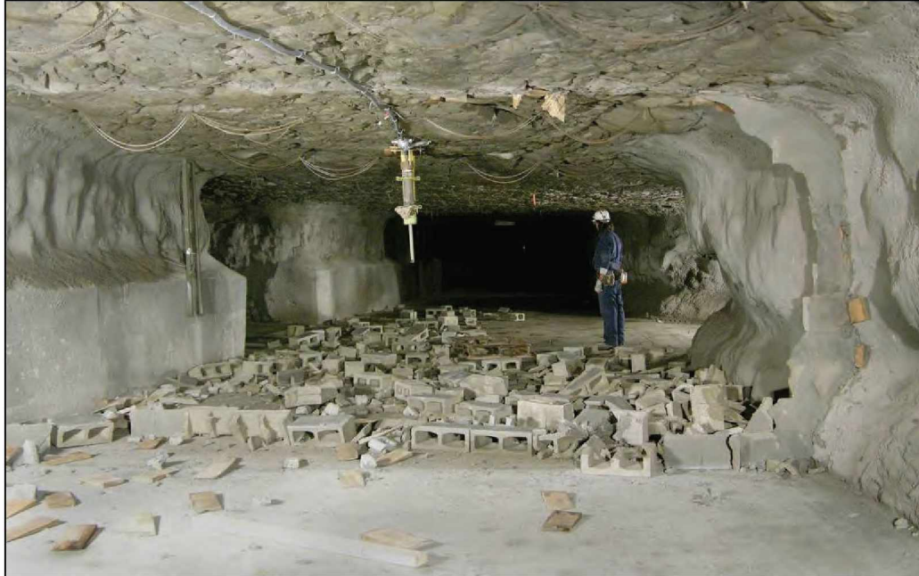
Figure 89.—Debris from the dry-stacked hollow-core concrete block stopping across B-drift after LLEM test #497.
