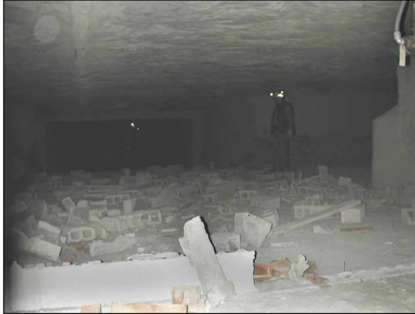
Figure 34.—Debris from dry-stacked hollow-core concrete block stopping in X-4 after LLEM test #428, viewed from C-drift.
