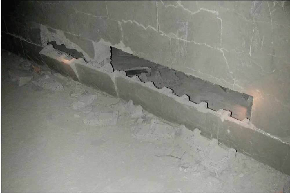
Figure 47.—Closeup of C-drift side X-6 dry-stacked hollow-core concrete block stopping after test #430, showing missing and damaged blocks.
