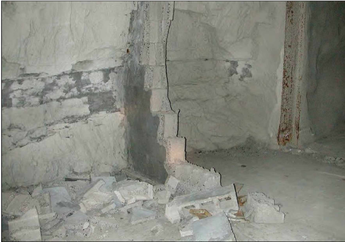
Figure 39.—Remnants of the dry-stacked hollow-core concrete block stopping in X-5 after LLEM test #428. The block shearing indicates roof-to-floor arching action.
