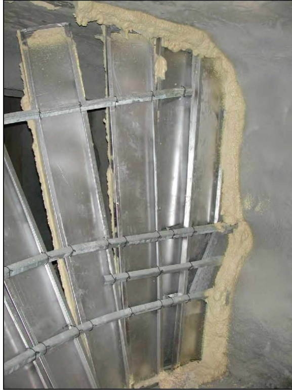
Figure 67.—Closeup of steel panel stopping still partially attached to outby rib in X-7 after LLEM test #458, viewed from B-drift.
