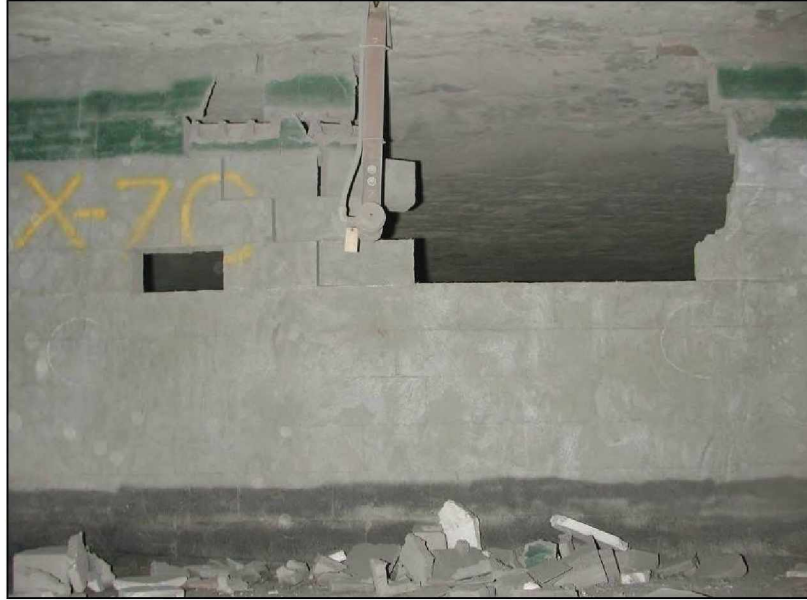
Figure 60.—Crosscut 7 dry-stacked hollow-core concrete block stopping viewed from C-drift after LLEM test #434.
