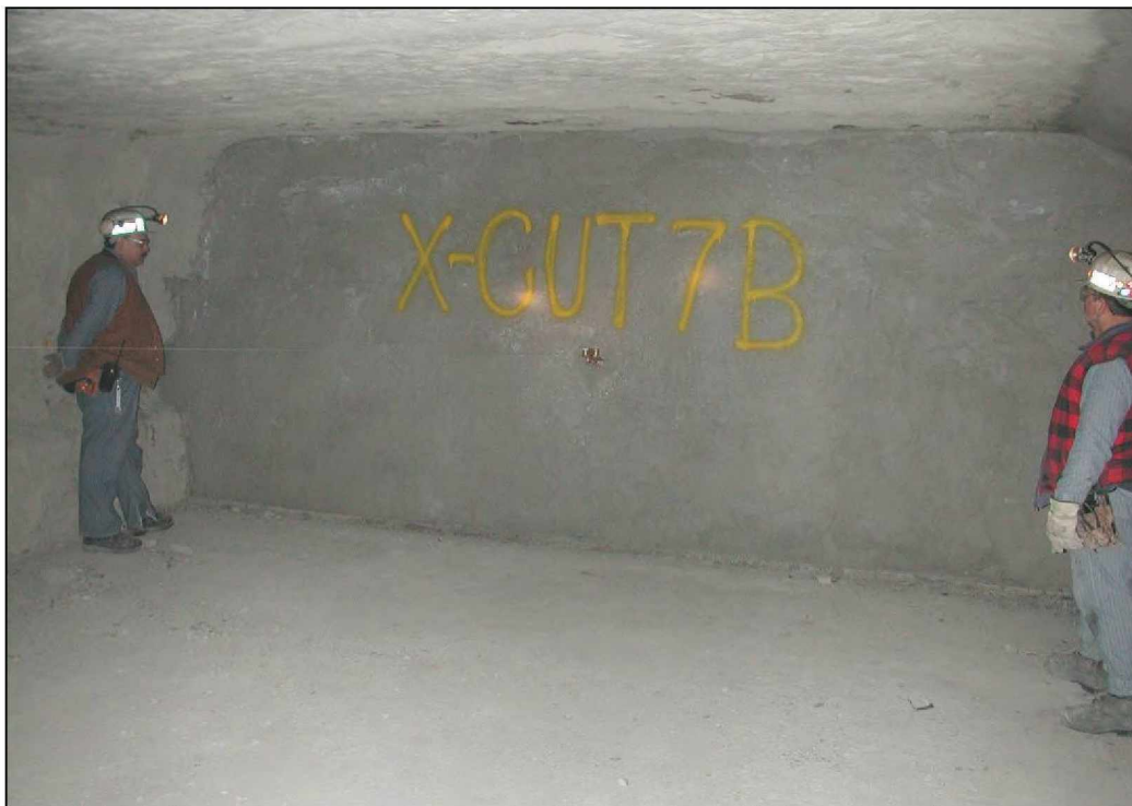
Figure 48.—The dry-stacked hollow-core concrete block stopping in X-7 remained intact after LLEM test #430.
