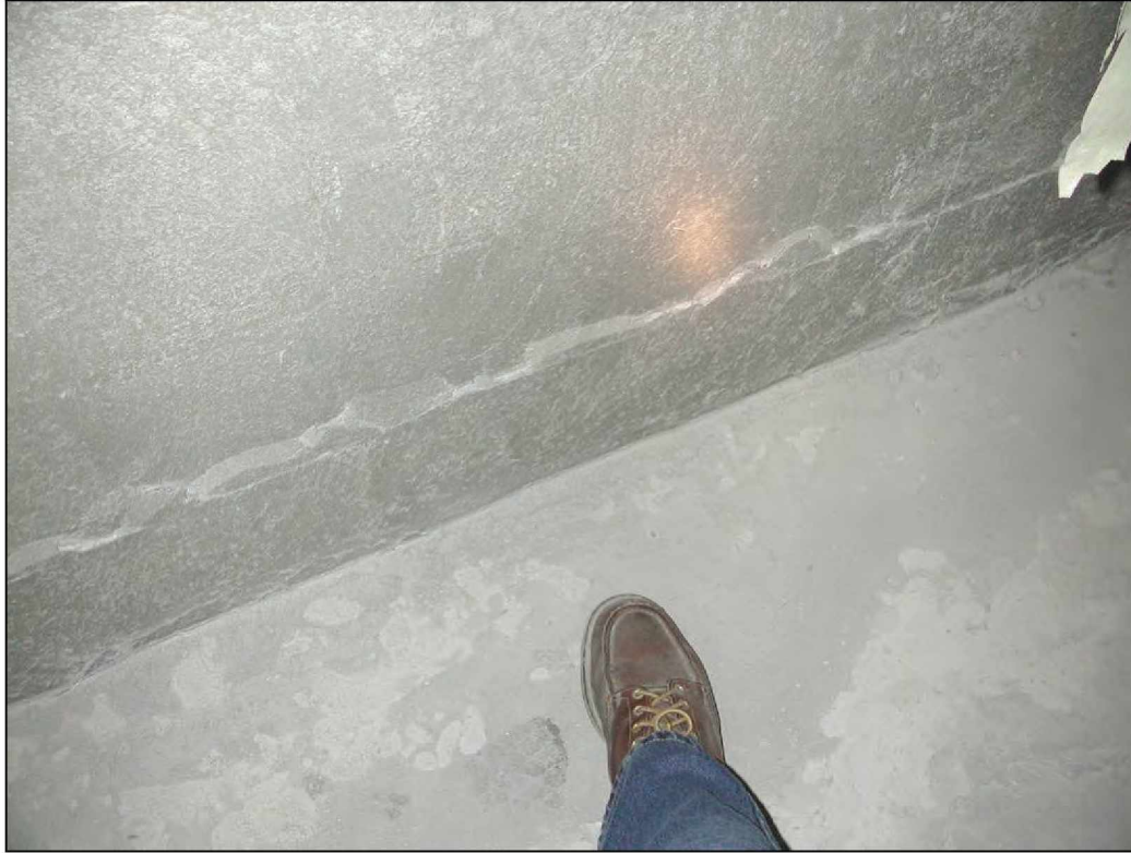
Figure 70. —Displacement of the second block course at the X-4 dry-stacked solid-concrete-block stopping after LLEM test #459, viewed from C-drift.
