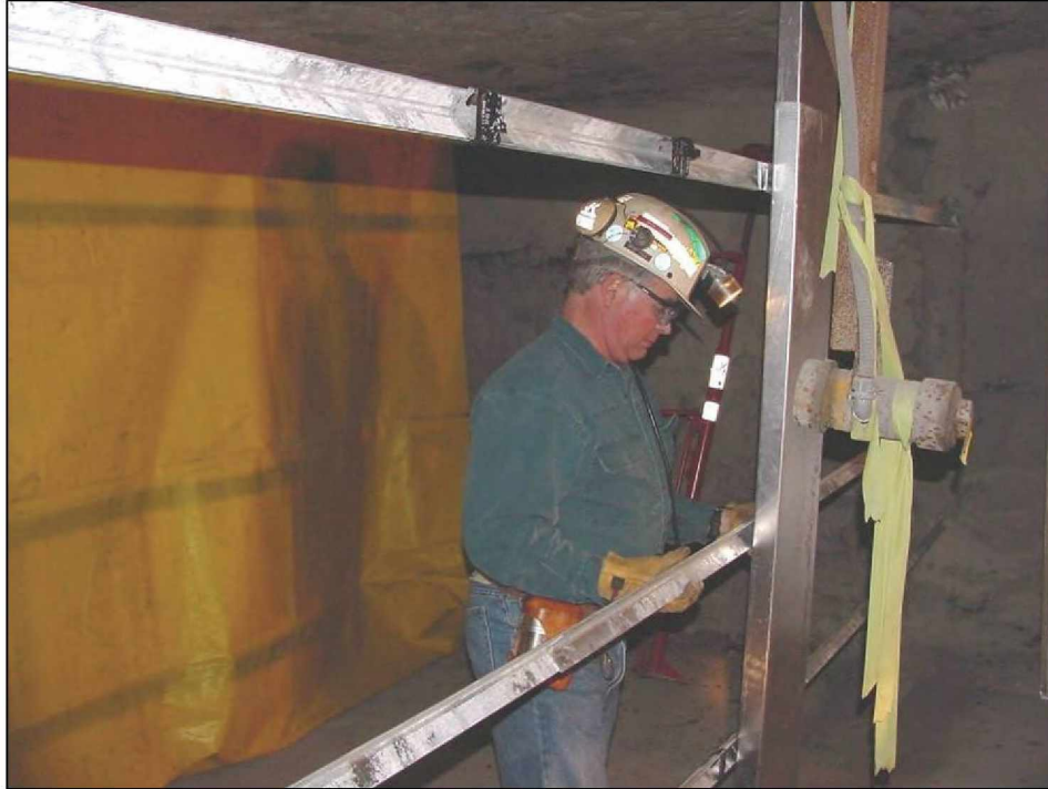
Figure 14.—Horizontal steel angles for attaching the steel stopping panels. The photo also shows the installed center panel.
