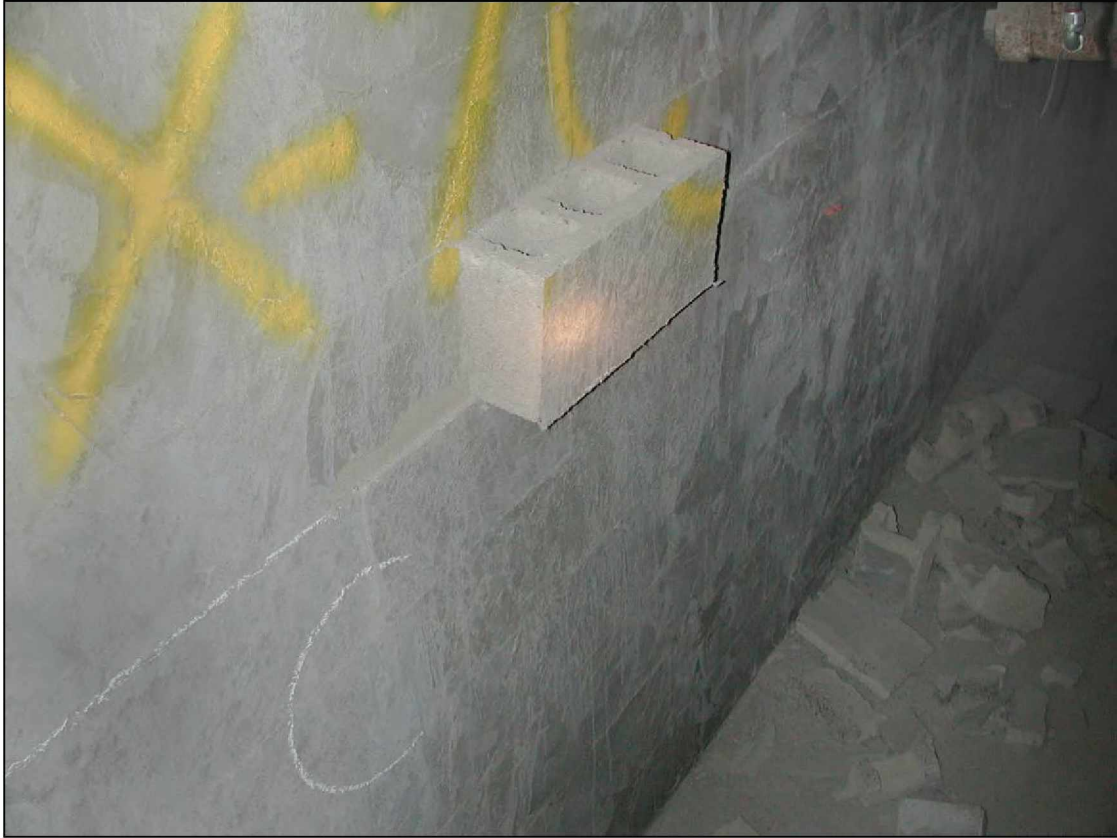
Figure 56.—Expanded view of hollow-core concrete block that is almost dislodged from X-7 dry-stacked stopping after explosion test #433.
