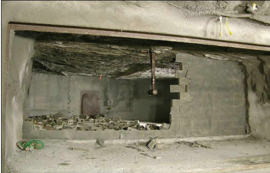
Figure 91.—Damage to the X-4 dry-stacked hollow-core concrete block stopping between B- and C-drifts after LLEM test #497.
