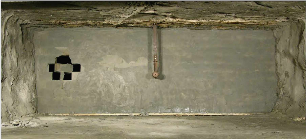
Figure 94.—Damage to the X-3 dry-stacked hollow-core concrete block stopping between B- and C-drifts after LLEM test #497.
