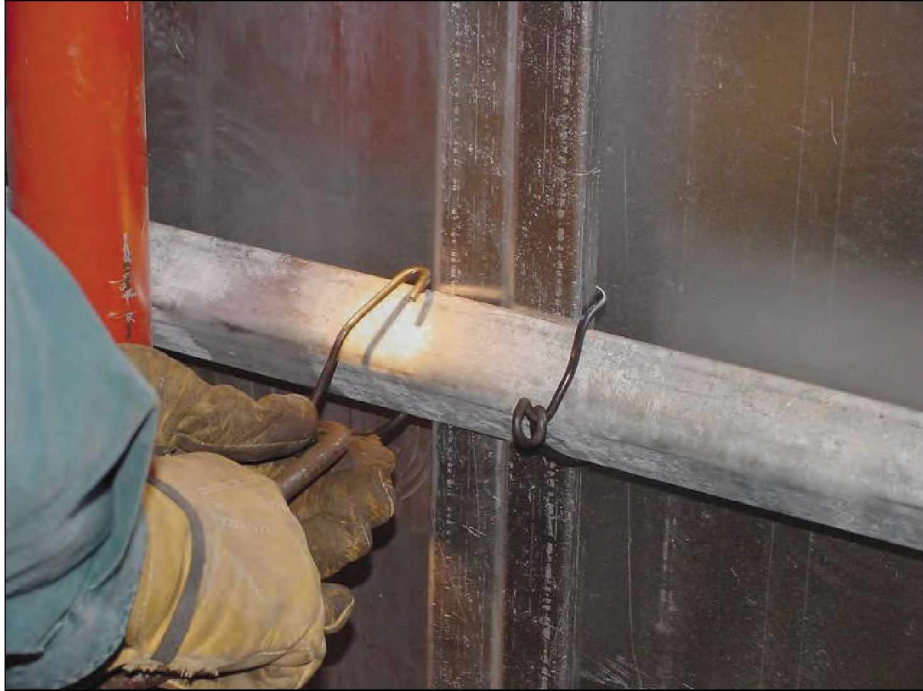
Figure 19.—Metal twist clamp used to secure open side of panel to the horizontal angle.
