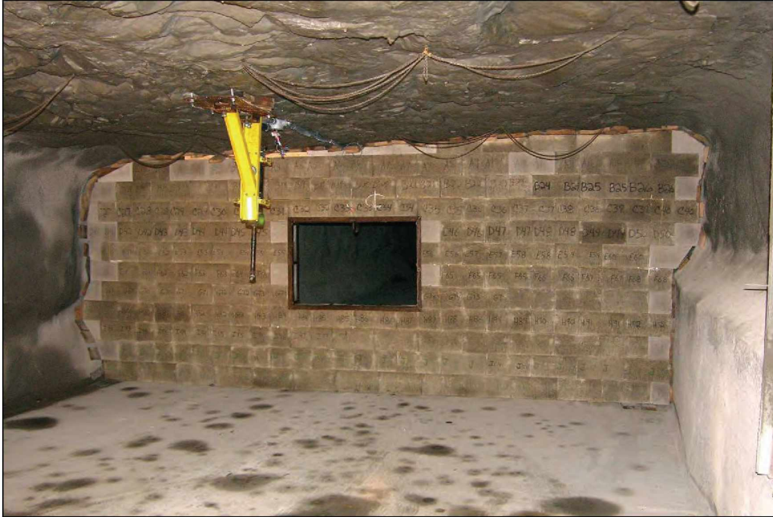
Figure 85.—Completed dry-stacked hollow-core concrete block stopping with simulated open regulator across B-drift.
