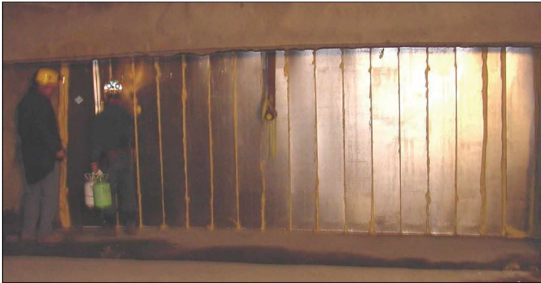
Figure 23.—Nearly completed steel panel stopping in X-6 showing closed, smooth panel sides facing C-drift.
