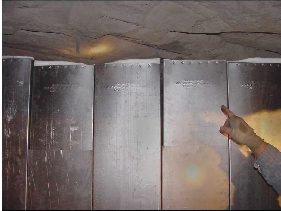
Figure 17.—Polystyrene foam head seal used to provide enhanced closure between metal panel and roof, as viewed from the C-drift side.
