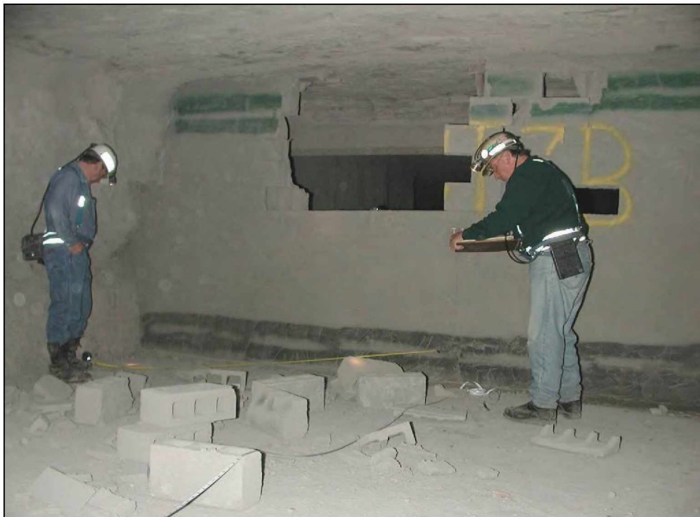
Figure 59.—Crosscut 7 dry-stacked hollow-core concrete block stopping viewed from B-drift after LLEM test #434.
