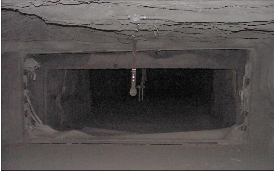
Figure 105.—Damage to the woven cloth stopping in X-6 after LLEM test #462.
