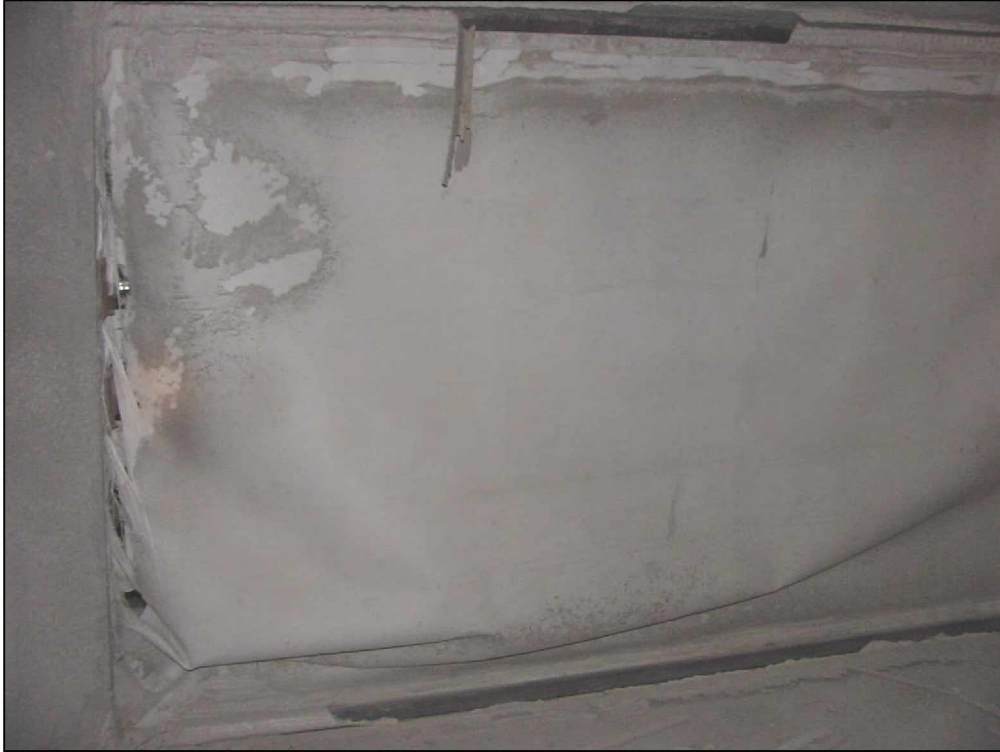
Figure 101.—Tears in the woven cloth on the outby rib of X-6 stopping after LLEM test #460, viewed from C-drift.
