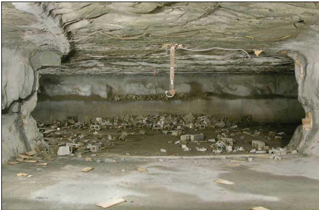
Figure 92.—Debris from the X-4 dry-stacked hollow-core concrete block stopping between A- and B-drifts after LLEM test #497.
