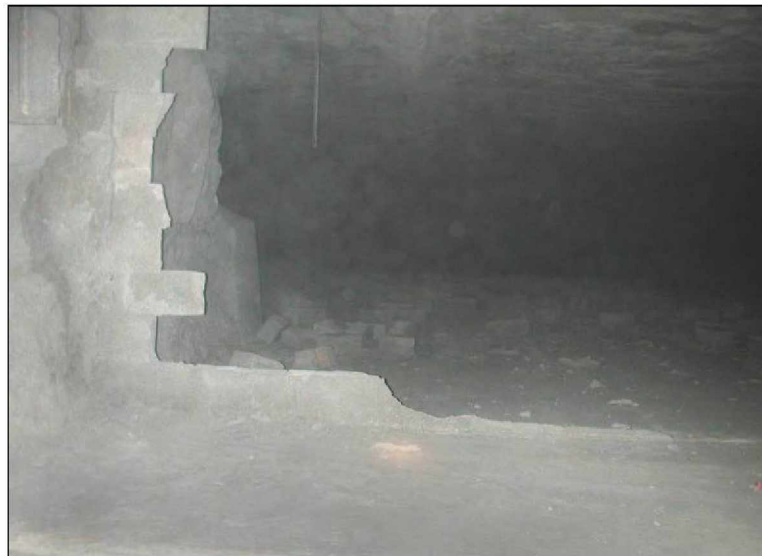
Figure 72.—Debris from the dry-stacked solid-concrete-block stopping and remaining blocks on the outby rib line in X-4 after LLEM test #462, viewed from C-drift.
