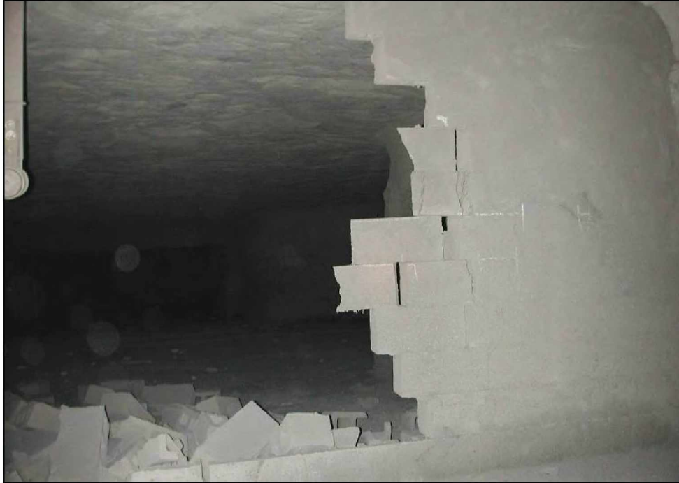
Figure 58.—Additional blocks partially dislodged from the right side of X-6 dry-stacked hollow-core concrete block stopping after test #434, viewed from C-drift.
