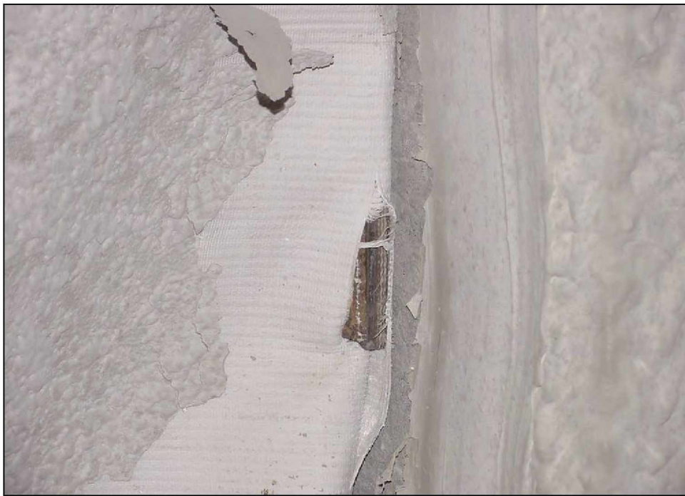
Figure 102.—Initial tear in the woven cloth at the corner steel roof bolt plate position on the inby rib of the X-7 stopping after LLEM test #460, viewed from C-drift.
