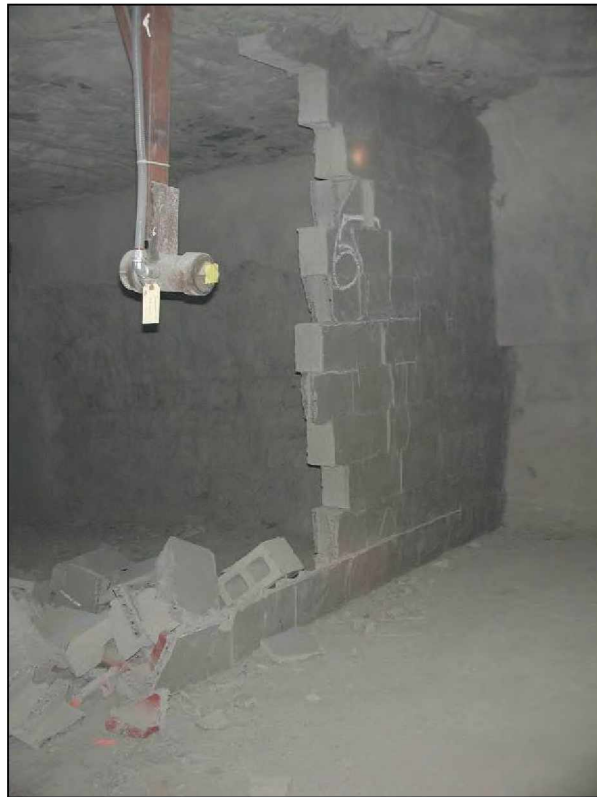
Figure 51.—Part of the inby side of X-6 dry-stacked hollow-core concrete block stopping remaining after LLEM test #433, viewed from C-drift.
