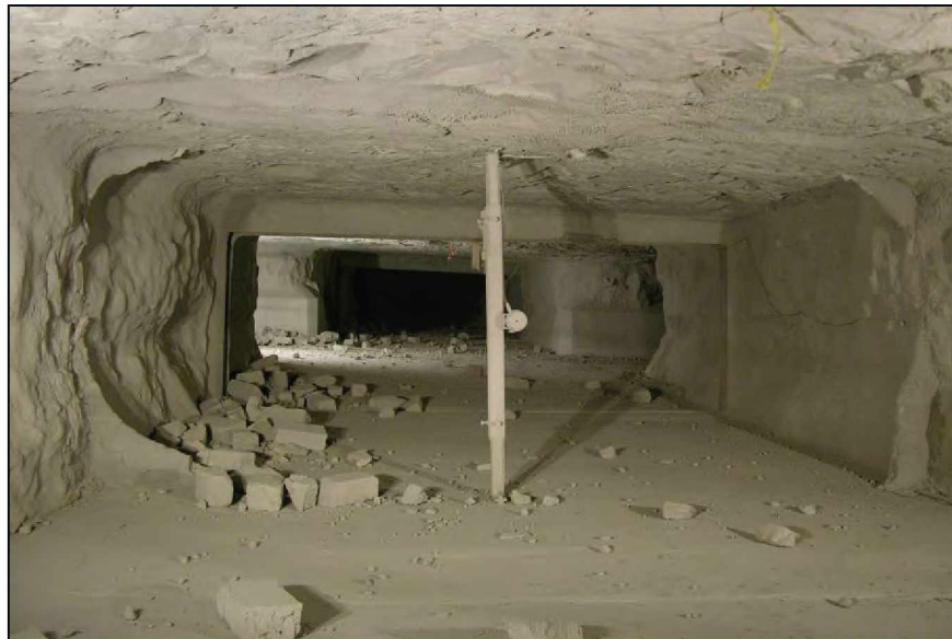
Figure 84.—Debris from 6-in (15-cm) thick, wet-laid solid block stopping in X-7 after LLEM test #519, viewed from A-drift.
