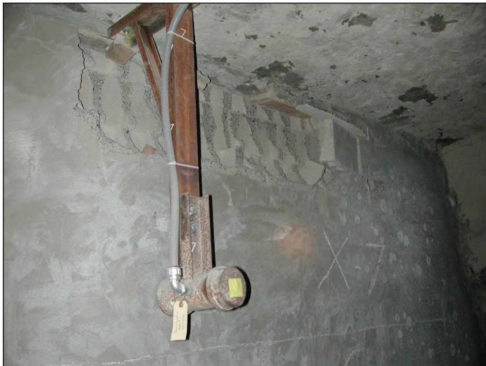
Figure 55.—Expanded view of top part of X-7 dry-stacked hollow-core concrete block stopping after explosion test #433, showing damaged blocks.
