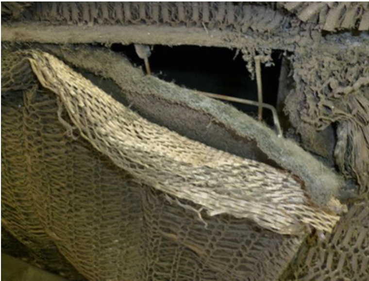
Figure 3. Damaged exhaust air filter in the spray paint booth. Photo by NIOSH.
