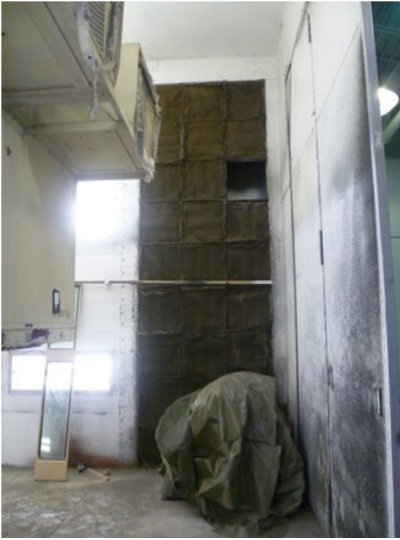
Figure 2. Missing exhaust air filters in the spray paint booth. Photo by NIOSH.
