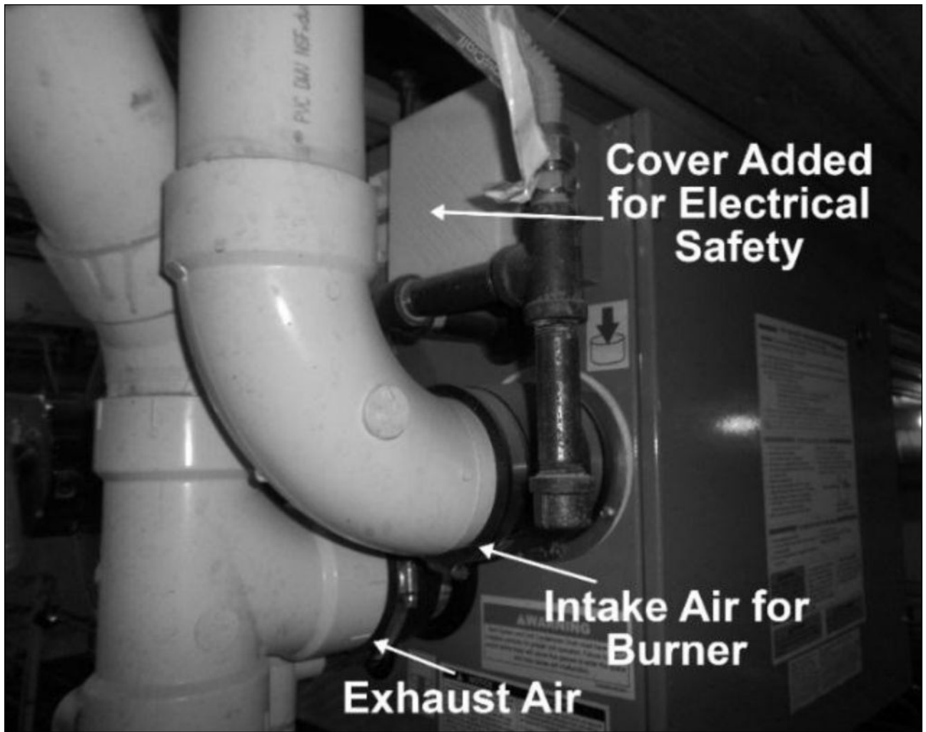
Figure 2. Back of installed vented heater, illustrating intake and exhaust ducts requiring installation.
