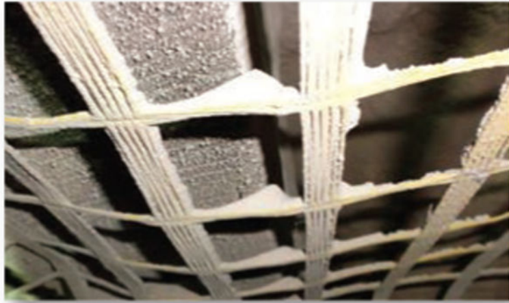
Figure 1. Indirectly applied rock dust is visible on the elevated surface of the mesh.
