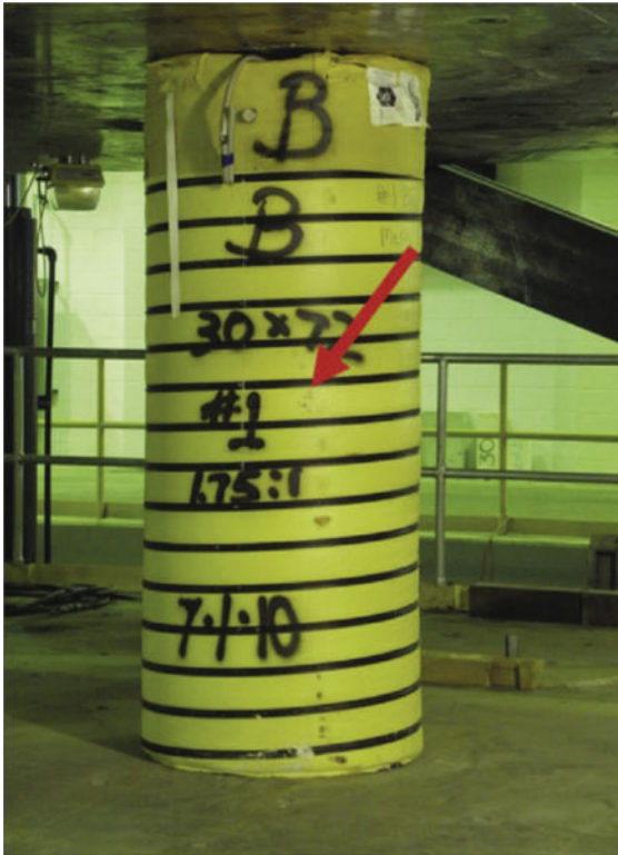
Fig. 16. Containment bag seam securing a metal reinforcement wire that is spiraled from the top to the bottom of the bag.
