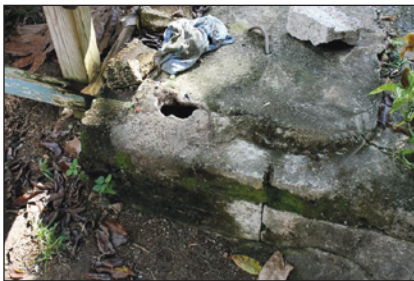
Broken septic tank cover
