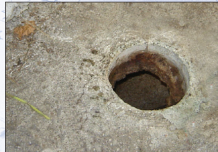
Open septic tank
