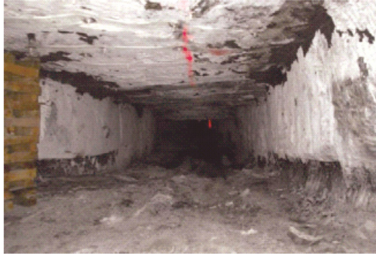
Fig. 5. Entry #1 panel L3 exhibiting poor conditions: floor heave, minor pillar spalling, and cutter roof.
