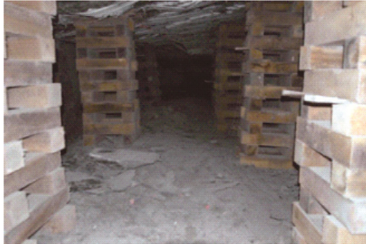
Fig. 4. Entry #5 panel L3 showing heavily cribbed area due to roof deterioration, pillar spalling, and floor heave, common to all panels observed.
