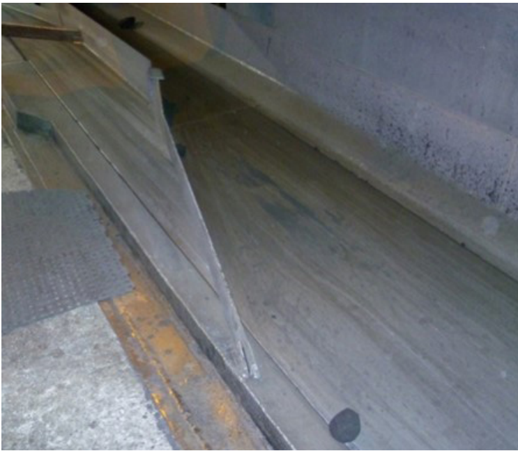
Figure 7. Casting diverter at the DISA 1 hot knockoff area. Photo by NIOSH.
