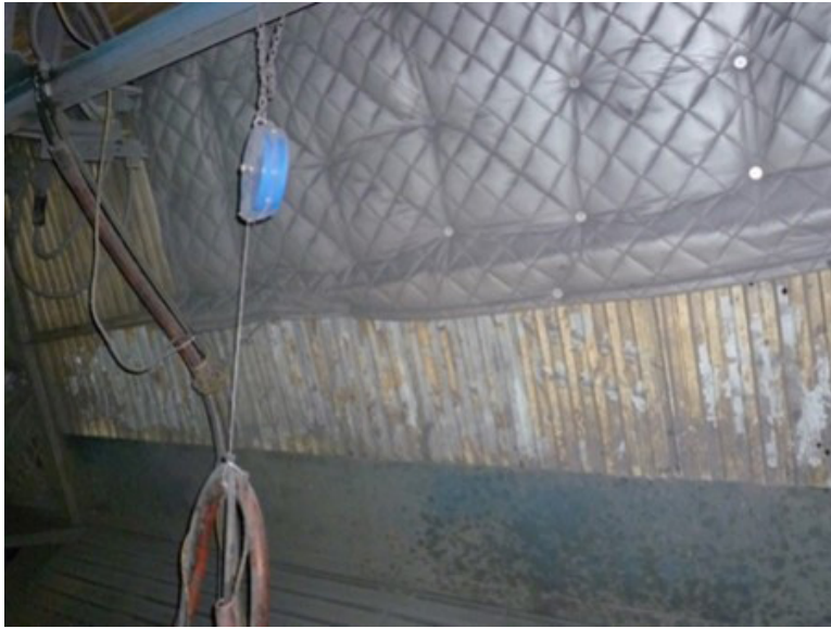
Figure 12. Knockoff area showing a corrugated metal wall partially covered with acoustic material. Photo by NIOSH.
