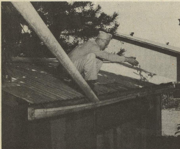
CLEARING A ROOF GUTTER BREEDING PLACE
