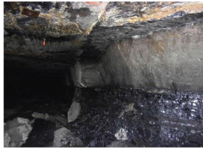
(b) Weak contact between the top section and immediate roof in mine USR 10
