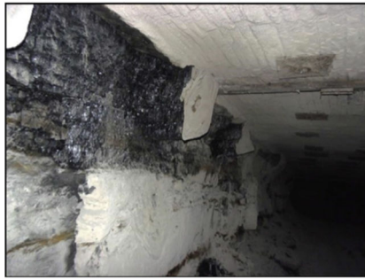
(a) Isolated rib bolts
