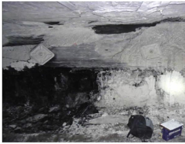
(a) Strong contact between the top section and immediate roof in mine SR 6
