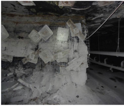
(a) 1.21 m straps of welded steel mesh at the pillar corner of mains, mine SR 5
