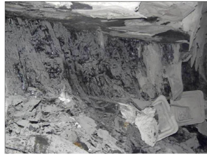
(b) Failed rib bolts
