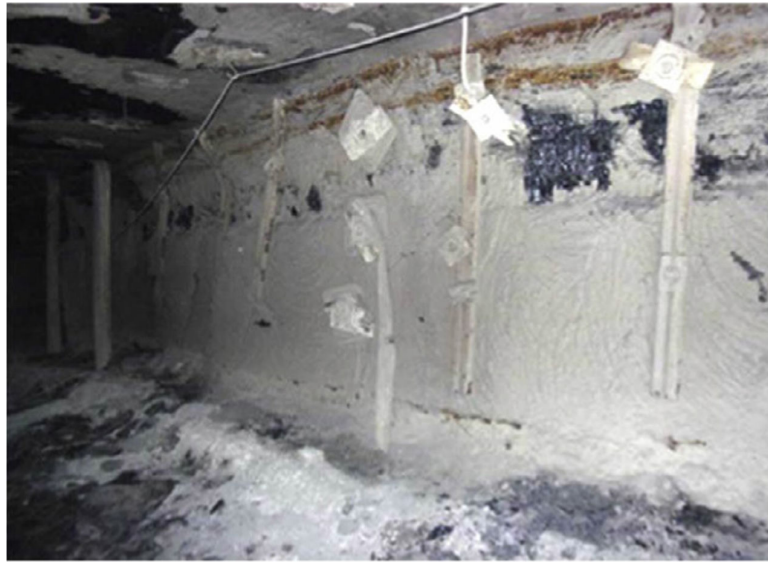
Fig. 9. Steel channels and timber props at SR 5 mine installed at an entry that exceeded the design width and height.
