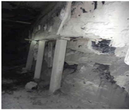
(a) Rib brow with spalling extended above the bottom row of rib bolts
