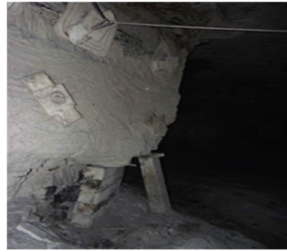
(b) Fractured brow at intersection
