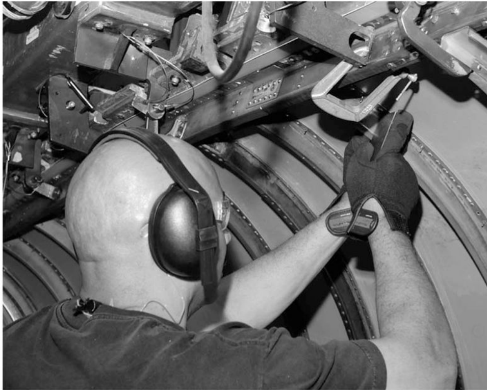
Fig. 6. A bucking bar operator provides the counter force at the backside of a rivet during a trial for Field Task 1. This process was similar for the other two tasks in the field assessment.
