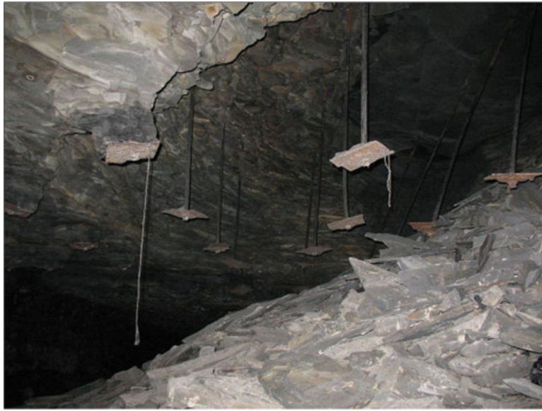
Fig. 11. Photograph showing how moisture-sensitive rock unraveled between bolts and fell to the ground
