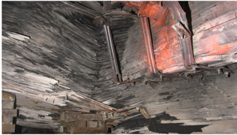
Fig. 5. Cutter roof failure of a weak shale rock at the roof-rib intersection
