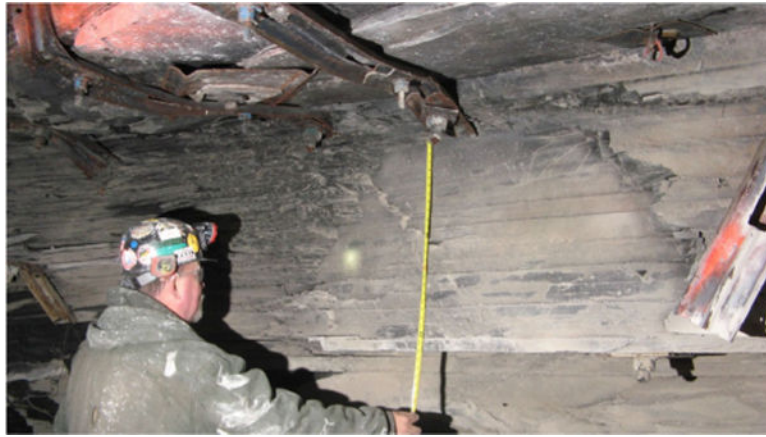
Fig. 2. Photograph showing a shale mine roof with thin beds
