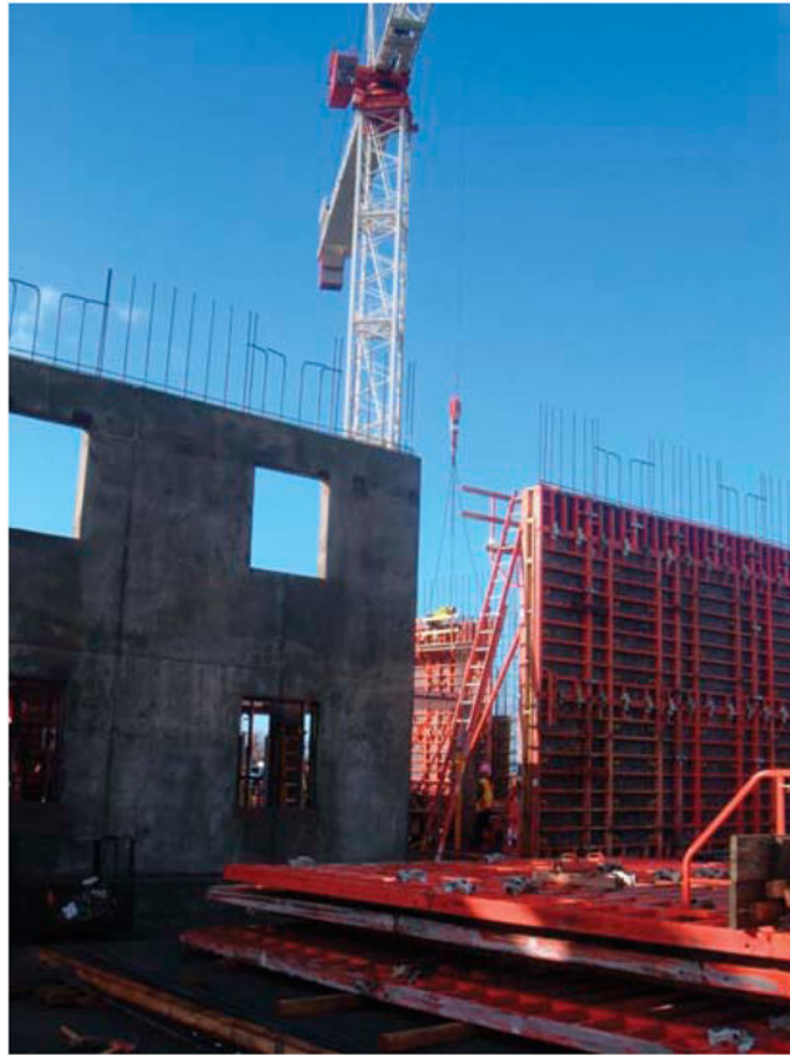
Photo 2. Use of a prefabricated formwork system (Photo 2) can lead to improve safety on construction sites
