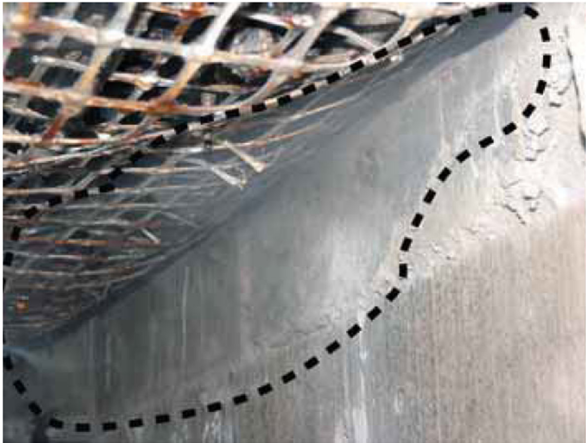
Figure 3. Smoke leaking through the stopping perimeter at the roof for Test 2
