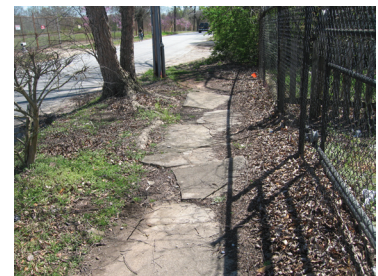
A lot (cracks and heaves)
