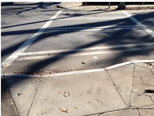
Curb cut (with NO tactile paving) Paving/truncated dome)
