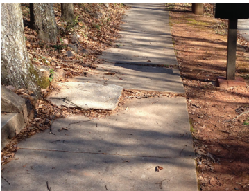
One (heave and cracks in sidewalk)
