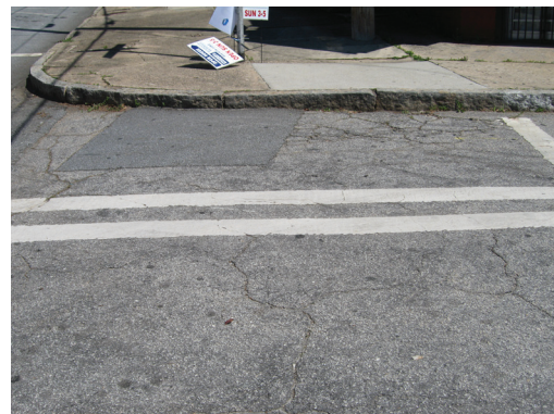
Crossing with no curb cutdome)
