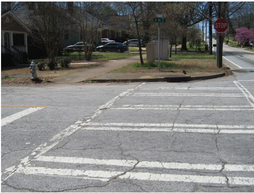
Ramp does not line up with crossing
