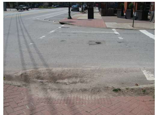
Faded or worn crosswalk marking
