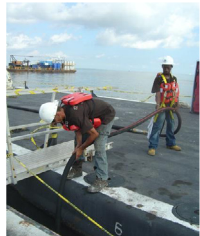
Figure 1. Workers using a vacuum hose to remove potential oil contaminated plant material from the water surface
