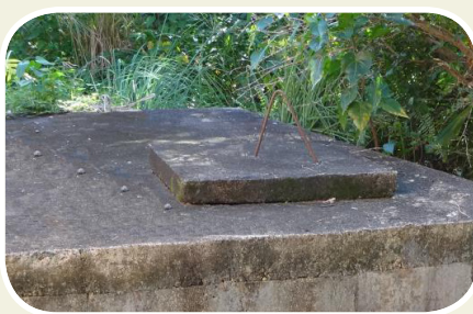
Septic tank with concrete cover
