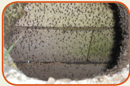
Mosquitoes in a septic tank
