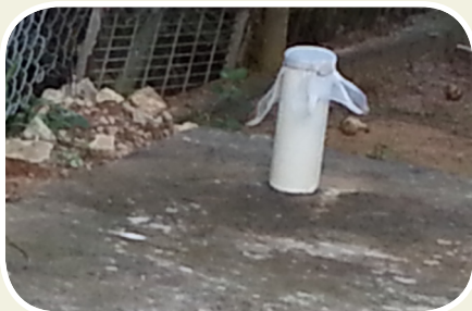
Septic tank ventilation pipe with screen mesh
