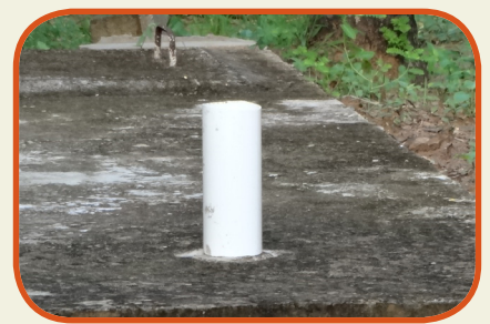
Cover ventilation pipes
