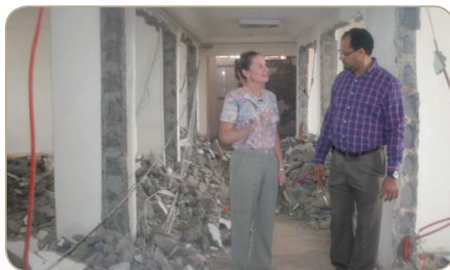
Dr. Martel discussing renovations for the expansion for the MoH's EOC in Guinea with Mark Hansey (CDC/OSTLIS/DPHDP).
