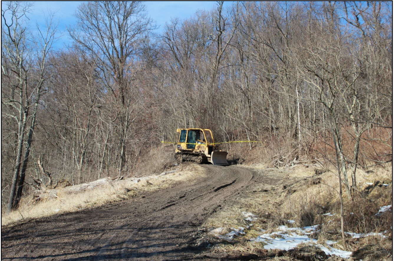
Photo 1. Road conditions up hill to cell tower collapse site. (Photo courtesy of WV State Police.)
