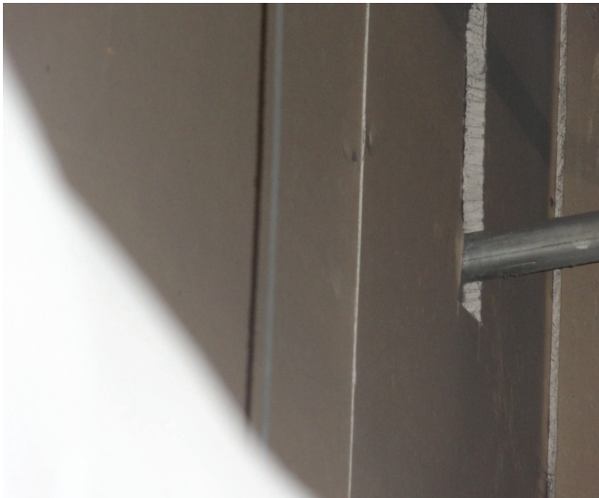
Figure 4. Hole between the firing ranges and showroom, above the ceiling. Photo by NIOSH.
