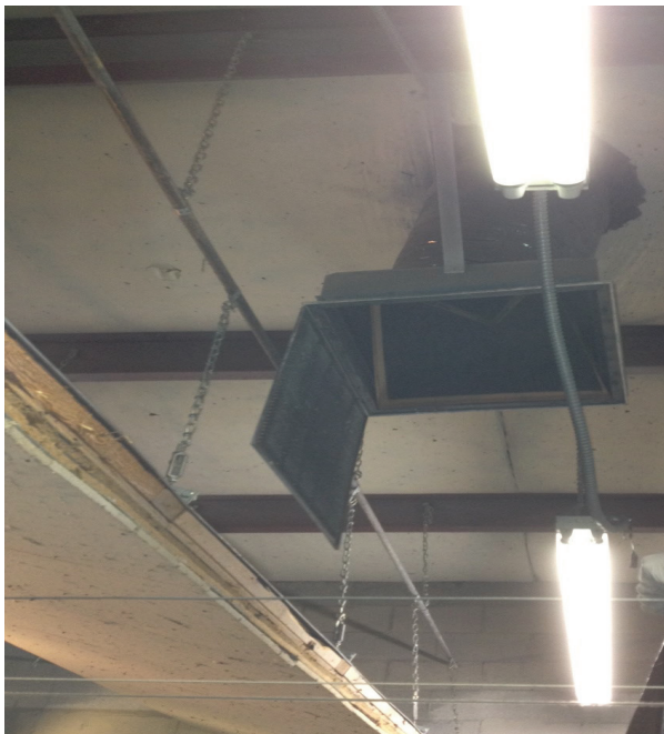
Figure 6. Dislodged, buckled air filter inside one exhaust outlet in range A. Photo by NIOSH.
