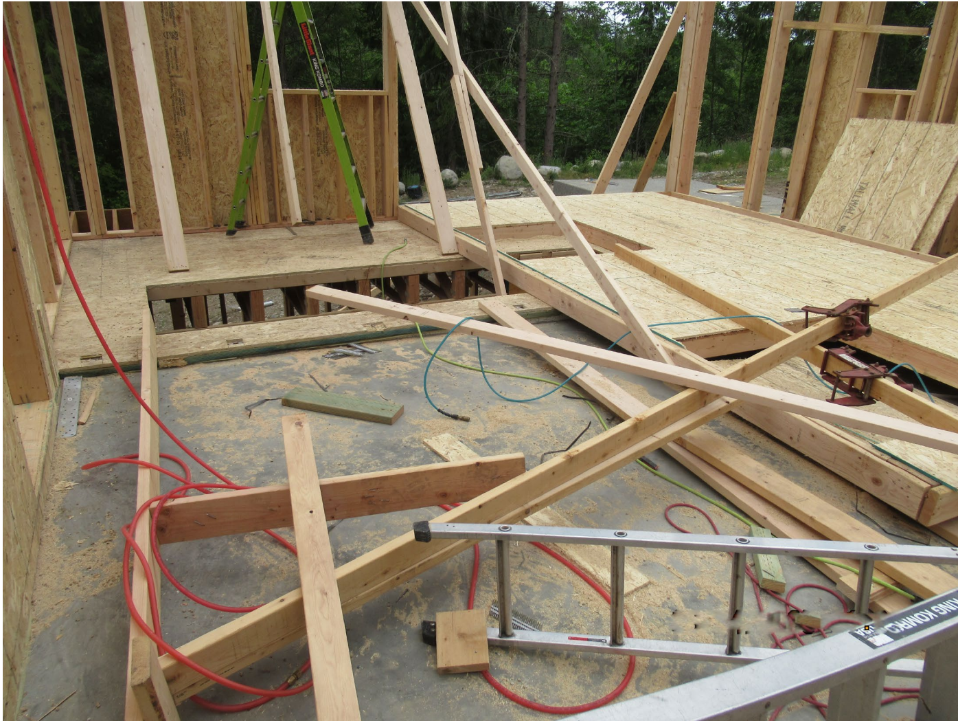
Image 7. Fallen wood bracing in work area where wall collapsed.
