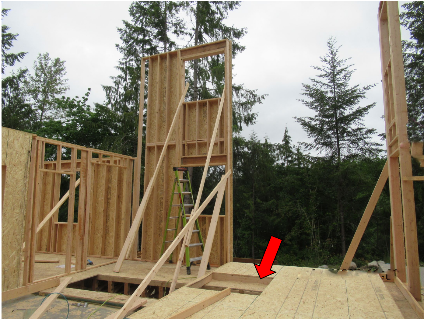
Image 5. Arrow shows approximately where framer was struck by wall and fell through opening.
