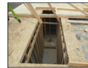
Unguarded floor opening.
