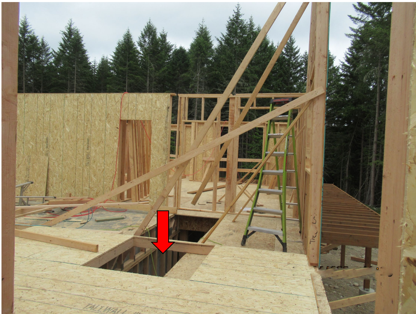
Image 6. Floor opening where framer fell.
