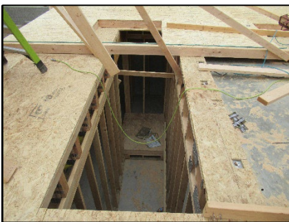
Unguarded floor opening.
