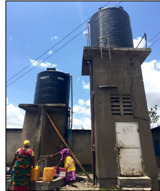
Figure 3: Water Storage Tanks
