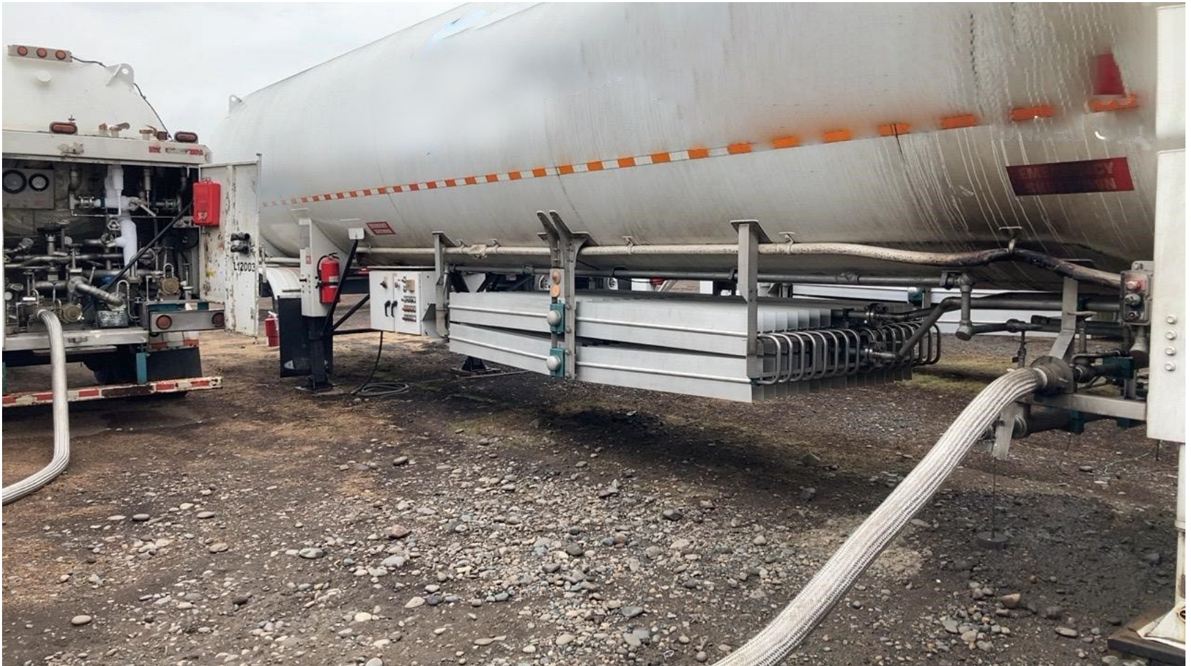
Image 5. Transport trailer on left and queen storage trailer on right with fire damage.
