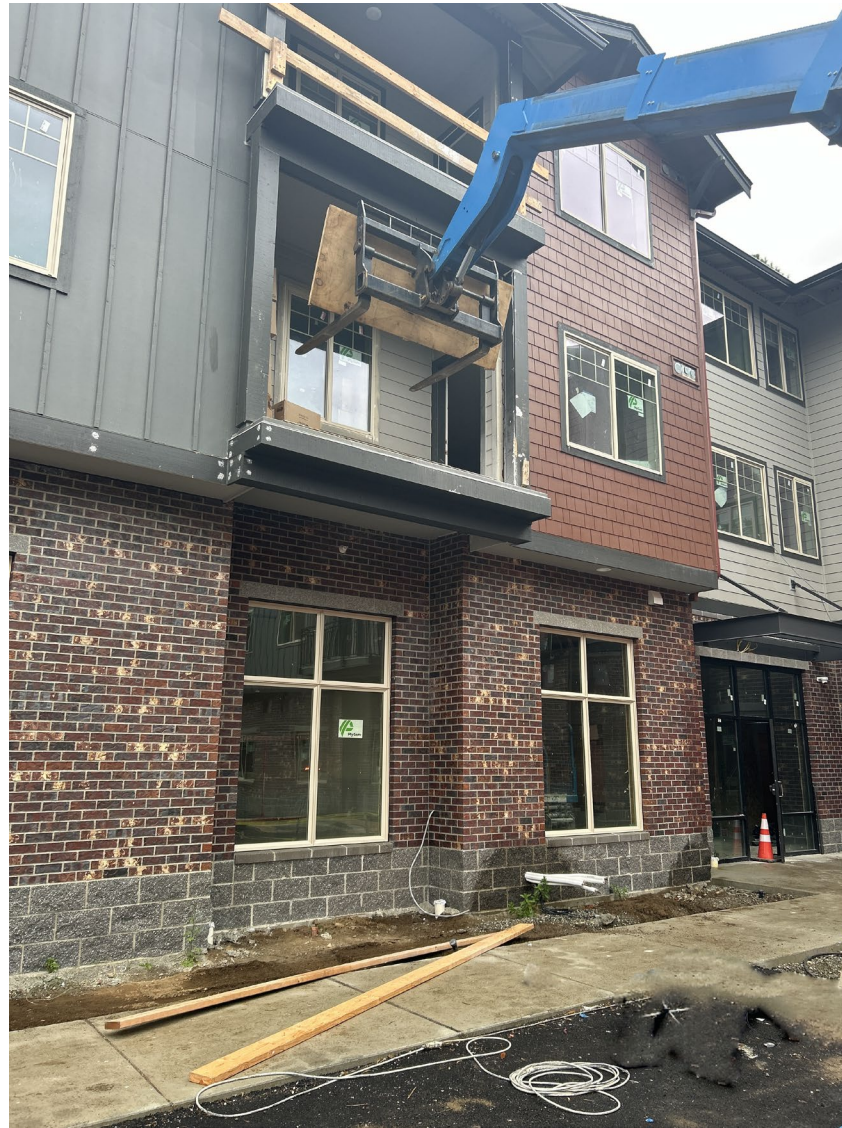
Image 2. Second-floor balcony where worker fell from, and failed guardrails on the sidewalk below.
