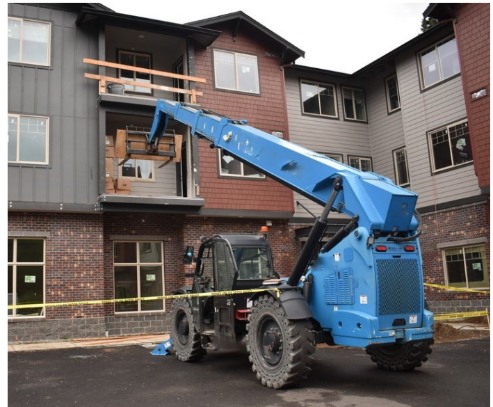
Image 1. Scene where worker fell.
