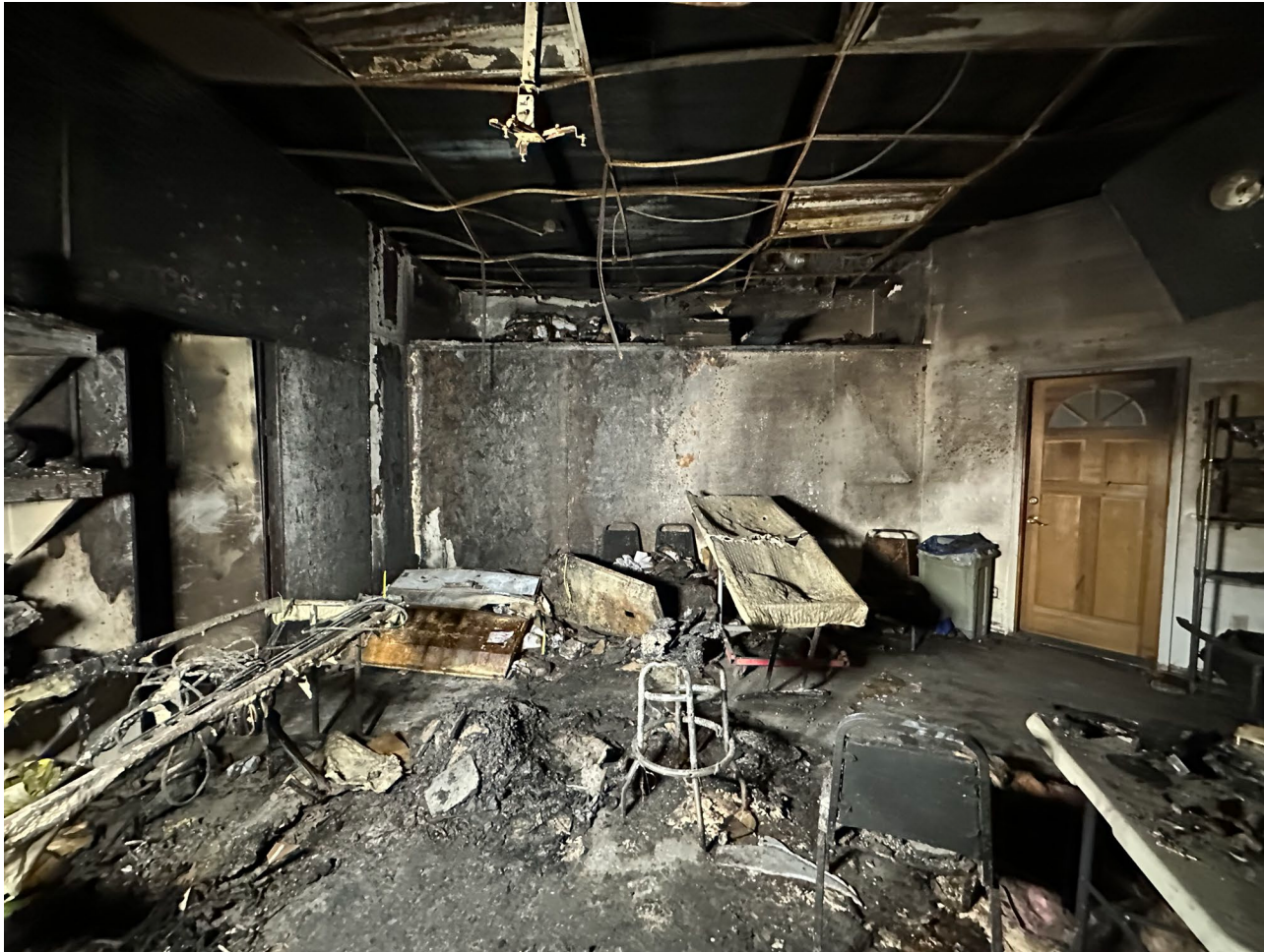
Image 4. Classroom where fire started and door to the instructor's workshop, lobby exit, and stairwell to first floor on the left.
