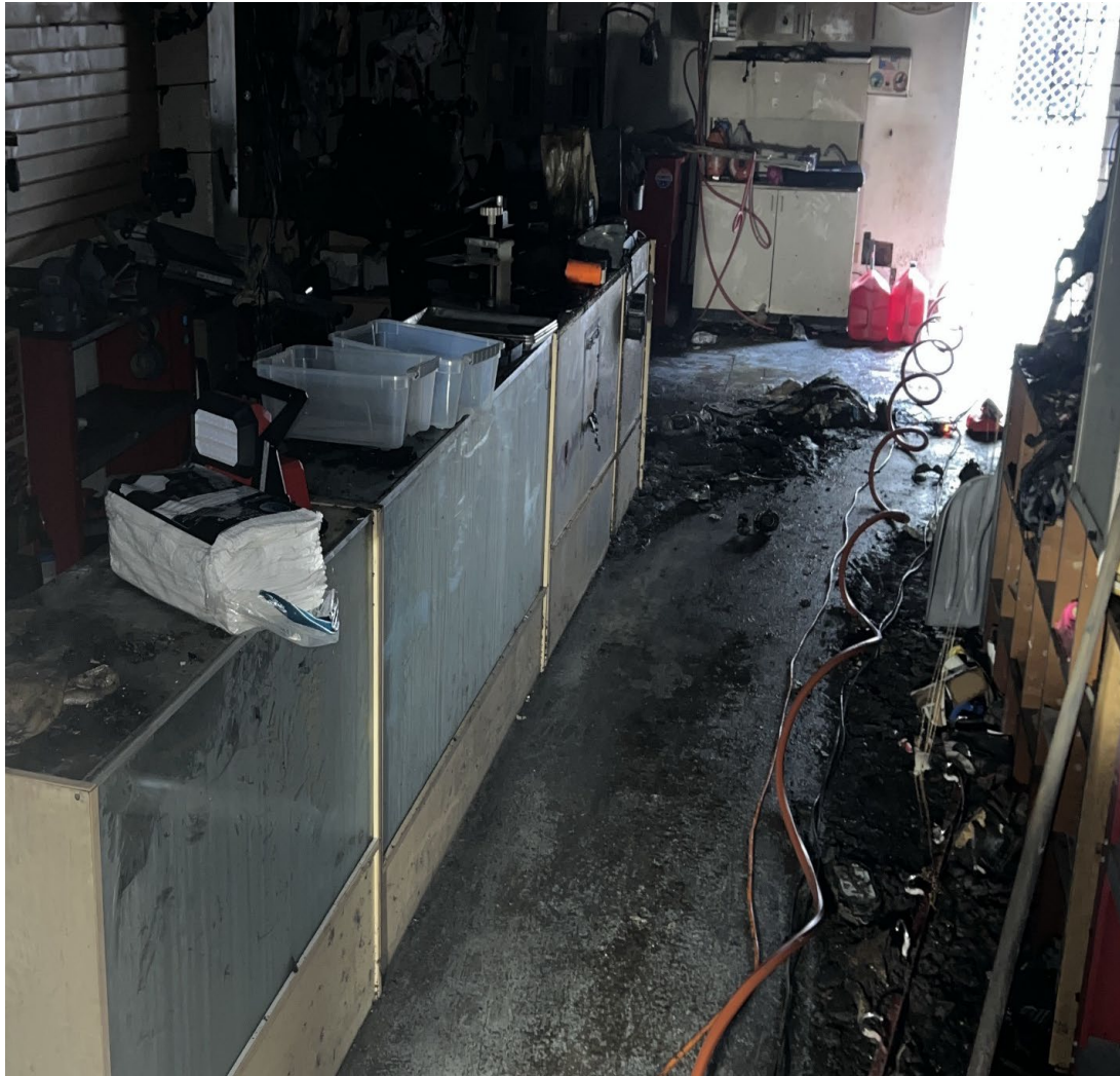
Image 2. Retail area in the second-floor lobby where one coworker was when the fire started and front exit the worker was blown out.
