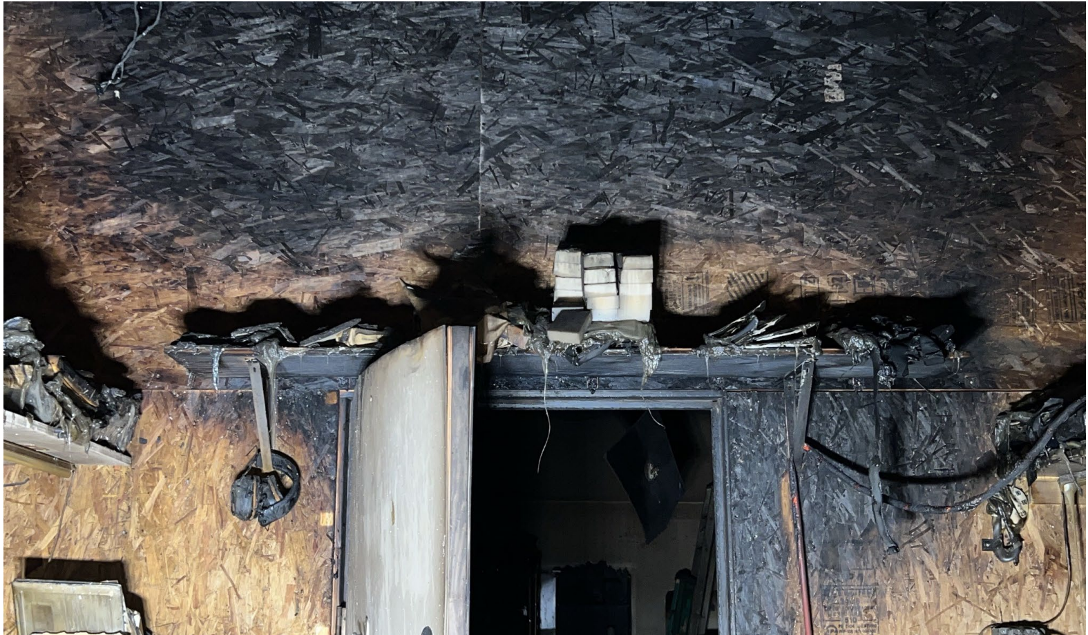
Image 9. Burn pattern on wall of workshop adjacent to classroom showing how the fire spread between rooms.
