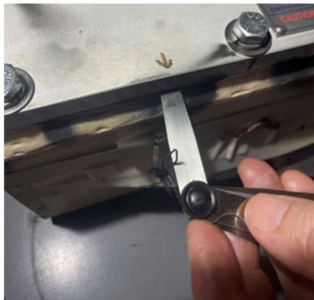
Fig. 10 A 0.004-inch feeler gauge penetrated the cover joint in several places after the thermal runaway test
