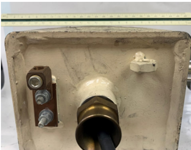
Fig. 12 Thermal runaway pressure deformed the XP enclosure bottom plate beyond allowable limits
