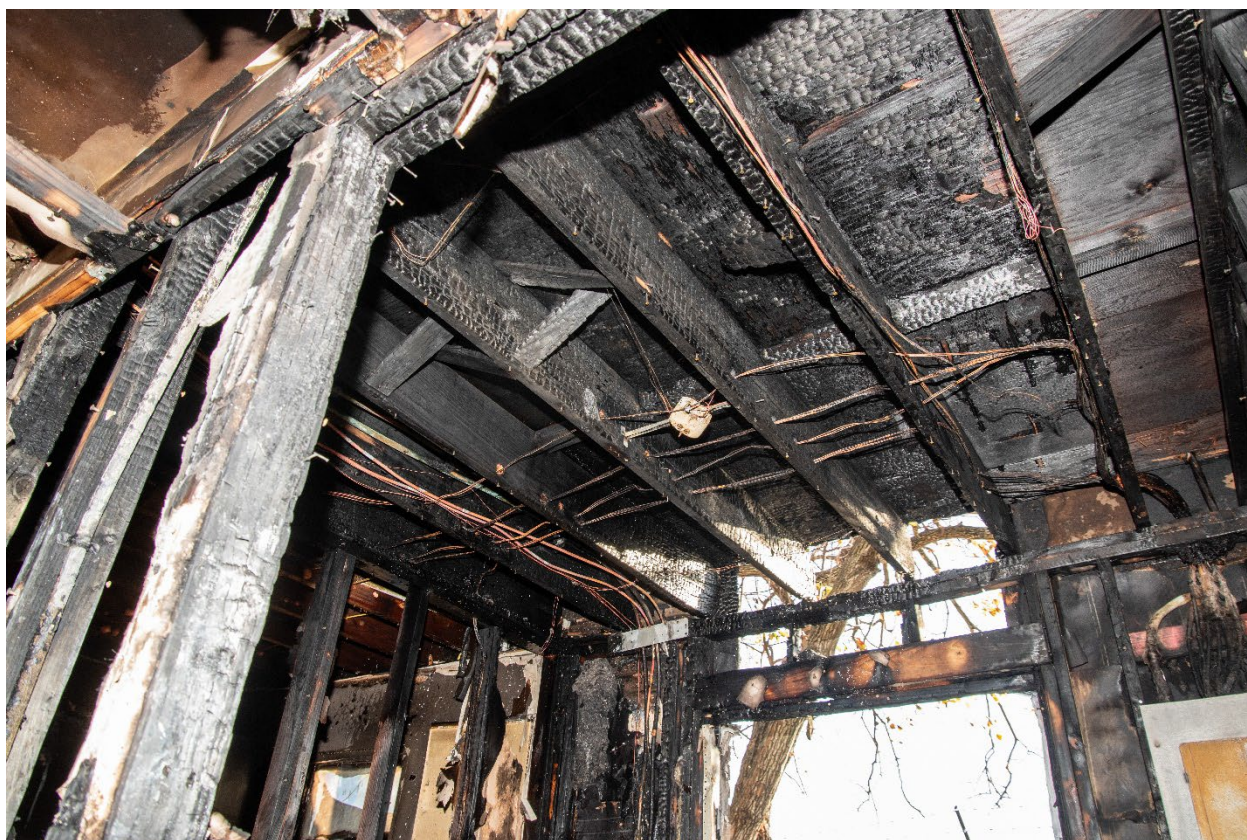
Photo 4: Detail of ceiling construction in bedroom 1. Charring and evidence of mass loss from the joists and bottom of the subfloor of division 2 are shown.
