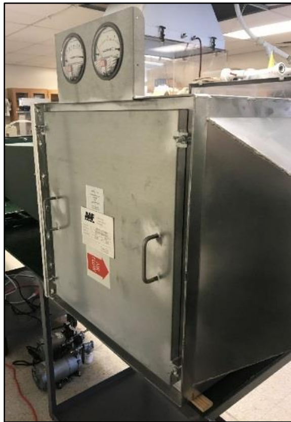
Figure 20: Wind Tunnel Exit Filter Housing.
