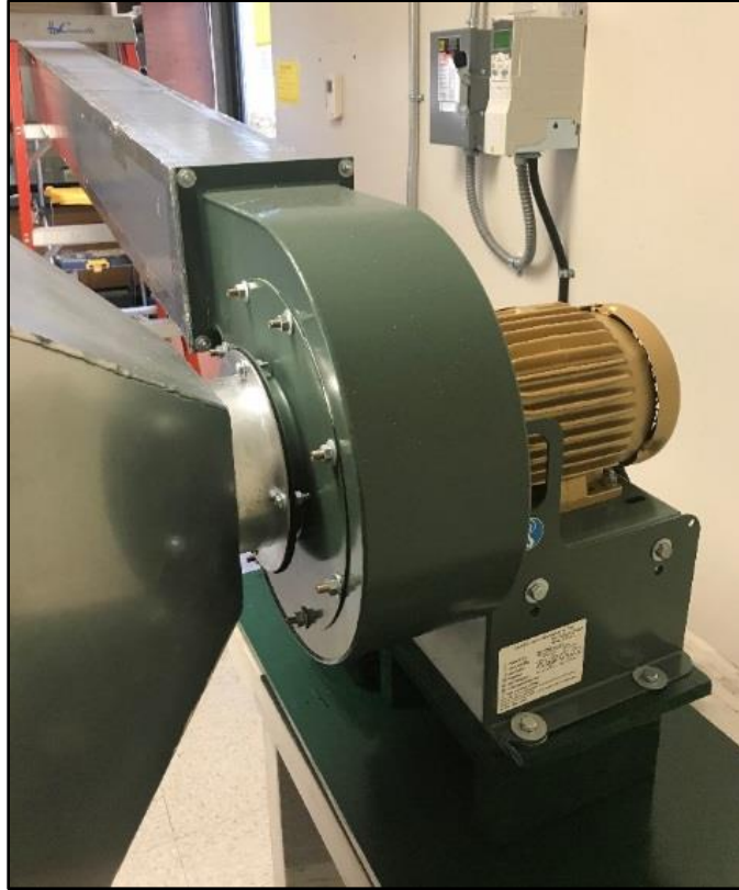
Figure 22: Wind Tunnel Fan, Motor, and Exhaust Duct.
