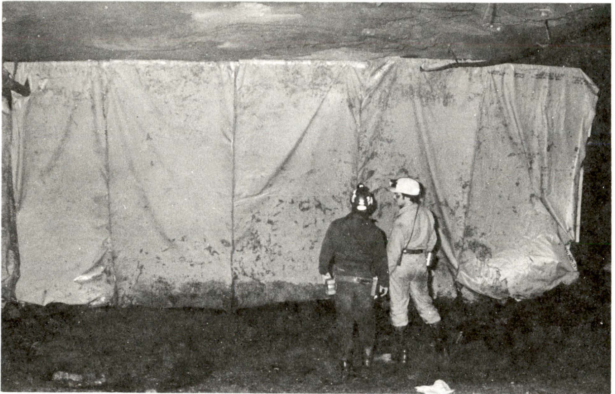
FIGURE 7. - Damage-resistant brattice at White Pine copper mine.
