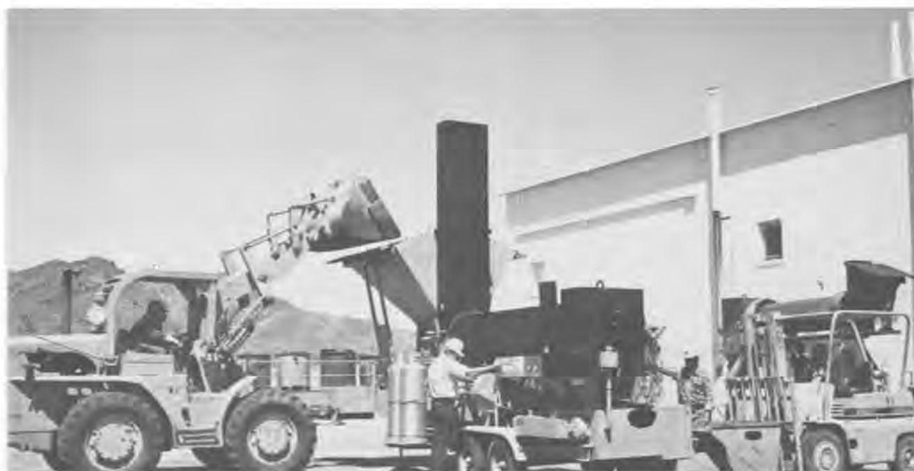
Figure 24.—Mobile 12-st/h SC mixing unit.
