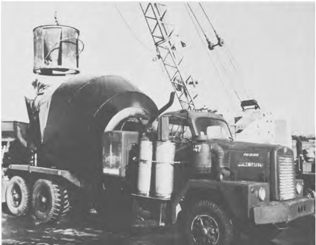
Figure 22.—Mobile mixing unit for SC.
