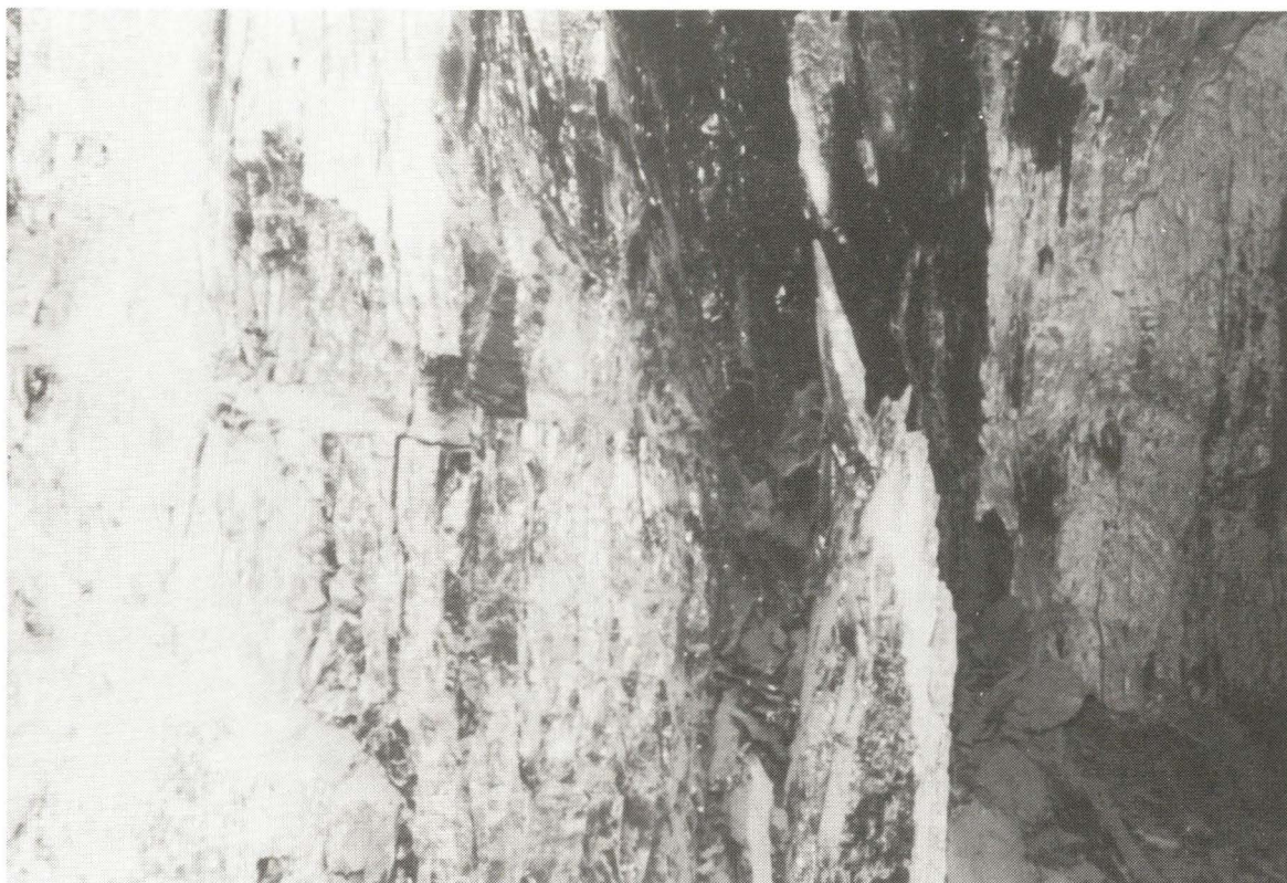
Figure 9.—Failure of zone D corner.
