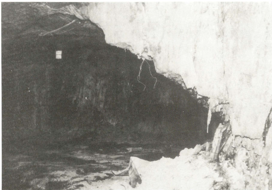
Figure 7.—Failure of zone B corner.
