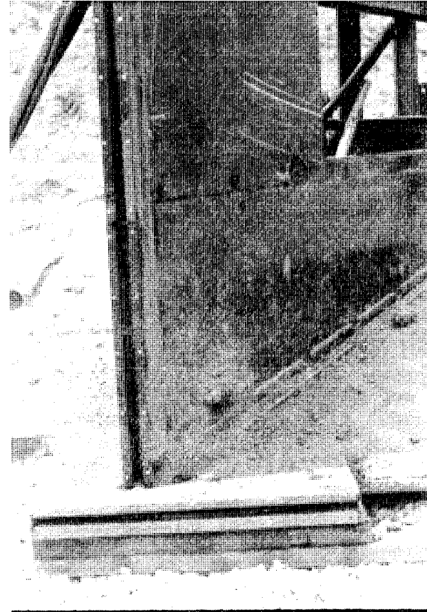
Figure 4.19. Weak construction with vertical wedge sitting on top of 3/8" plate.
