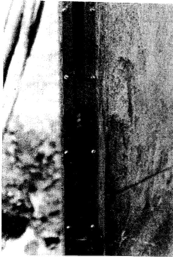
Figure 3.9. Initial design of slot guard as installed.
