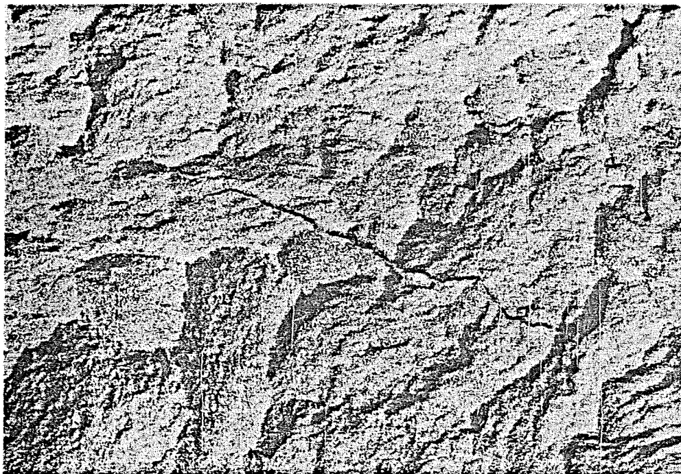
FIGURE 2-7. - Crack detail (open).
