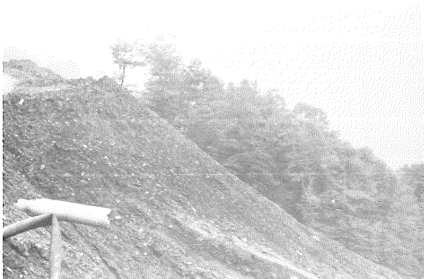
FIGURE 4 - Oversteepened Slope and Example of Inadequate Spillway Design
