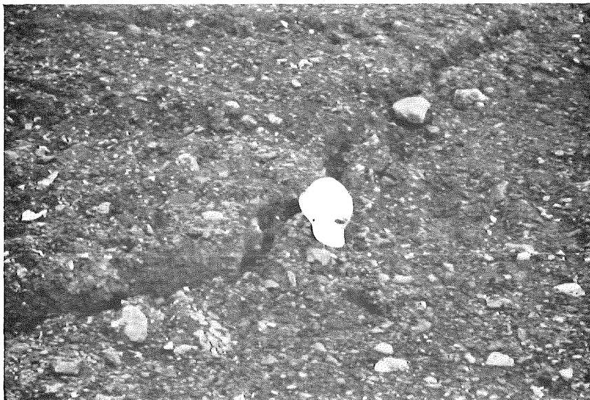
FIGURE 3 - Surface Crack in a Coal Refuse Embankment
