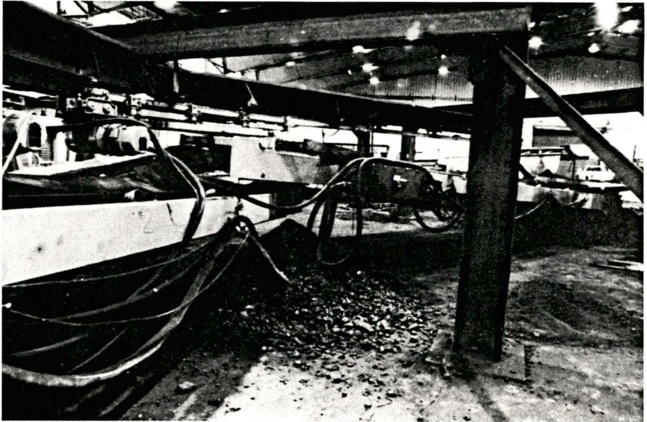
FIGURE 18. — Spillage under the inby intermediate transfer unit.
