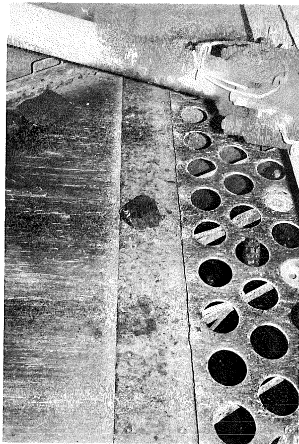
FIG. 29. GOODYEAR ARMAPLATE (1/2 in.) INSTALLED BETWEEN THE TAIL END OF PRIMARY SCREEN AND LEADING EDGE OF PICKING TABLE.
