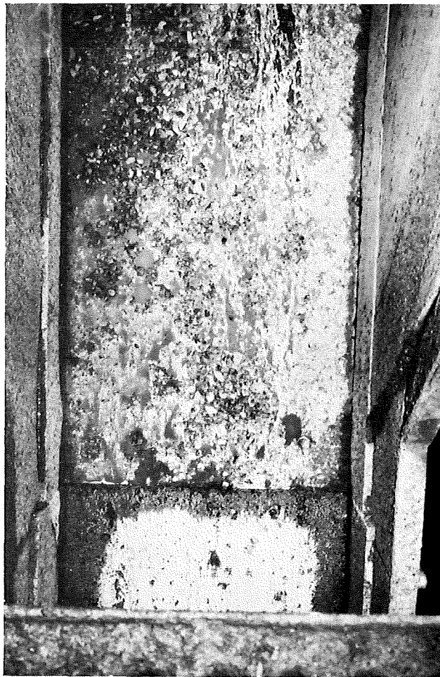
FIG. 70. URETHANE IMPACT PAD IN REFUSE DESANDING SHAKER DISCHARGE CHUTE.
