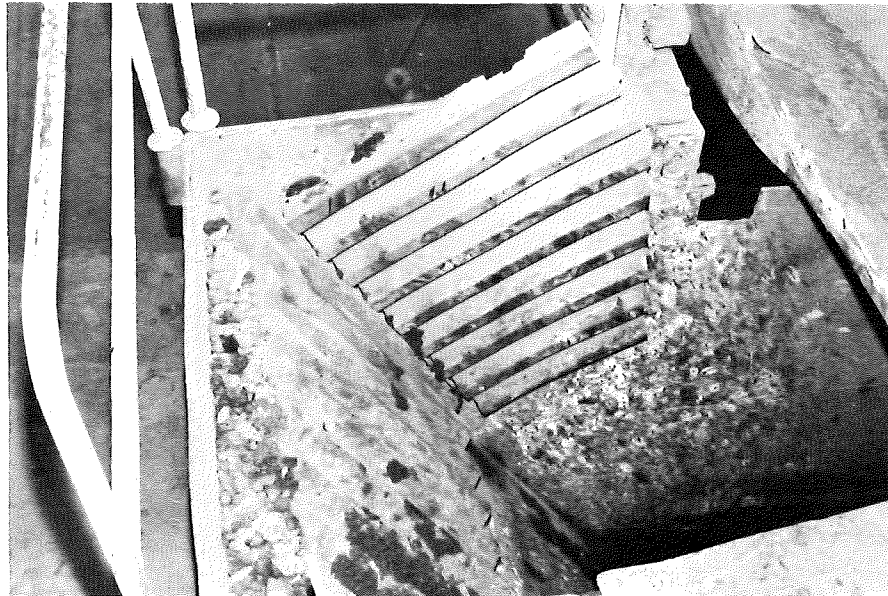
FIG. 31. PROFILED TRELLEBORG AT INFEED TO McLANAHAN ROCK CRUSHER.
