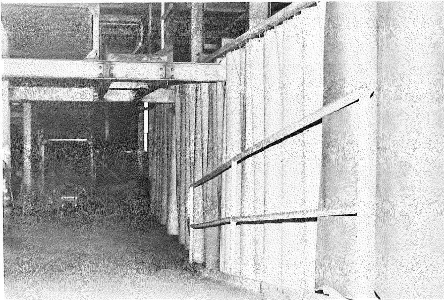
FIG. 56. CLEAN-COAL DESANDING SHAKER AREA AFTER INSTALLATION OF CURTAINS (LOOKING DOWN RAMP FROM BUILDING A).
