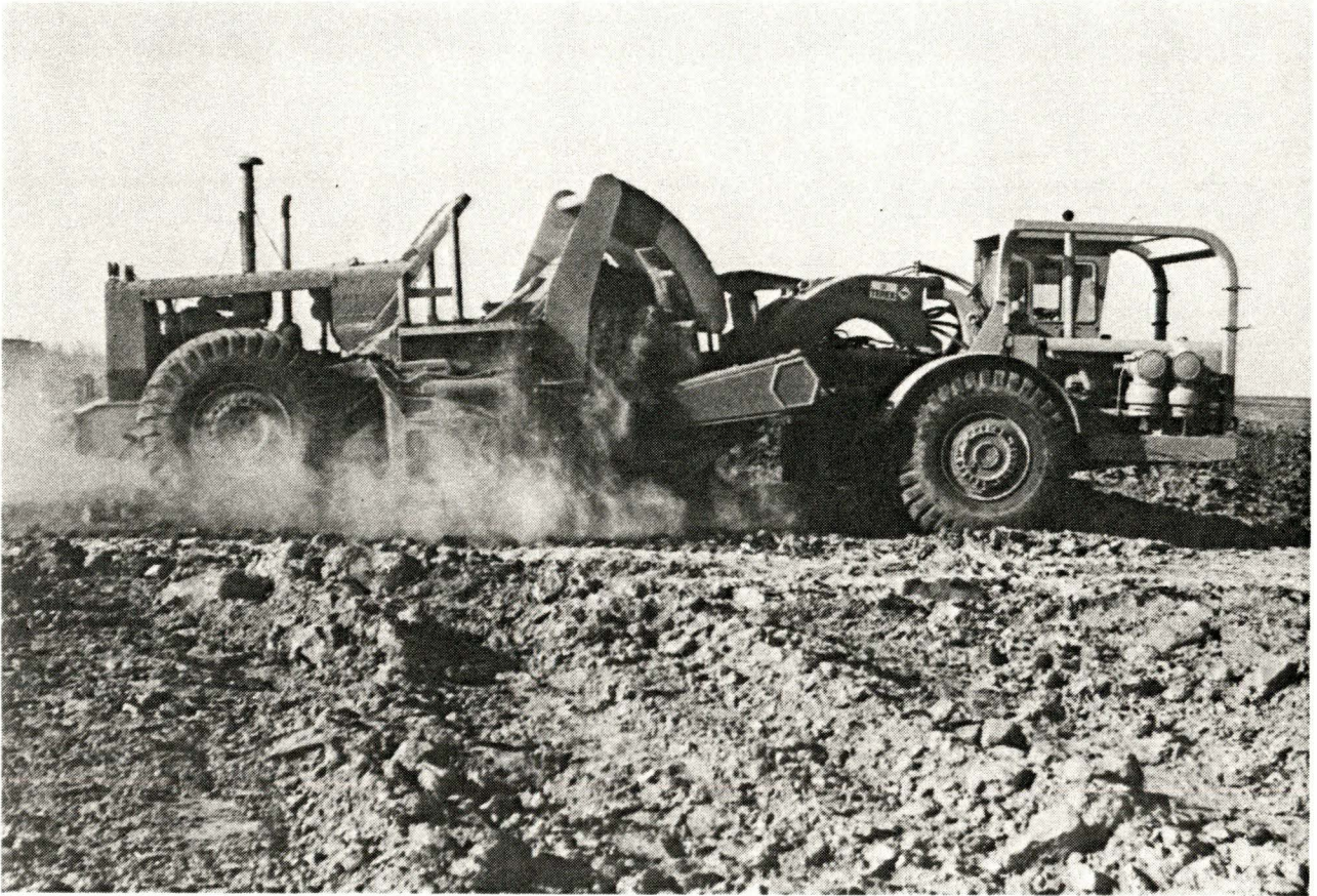
FIGURE 30. Scrapers Used for Both Topsoil and Subsoil Removal and Transport on the Power Mine
