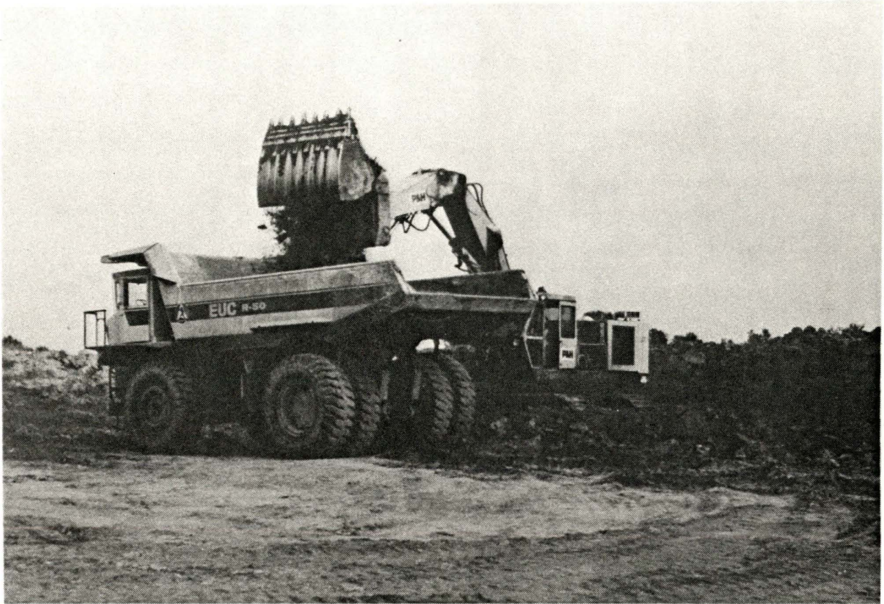
FIGURE 18. Rooting Medium Removal and Loading by Front Shovel/Truck System on the Brazil Mine
